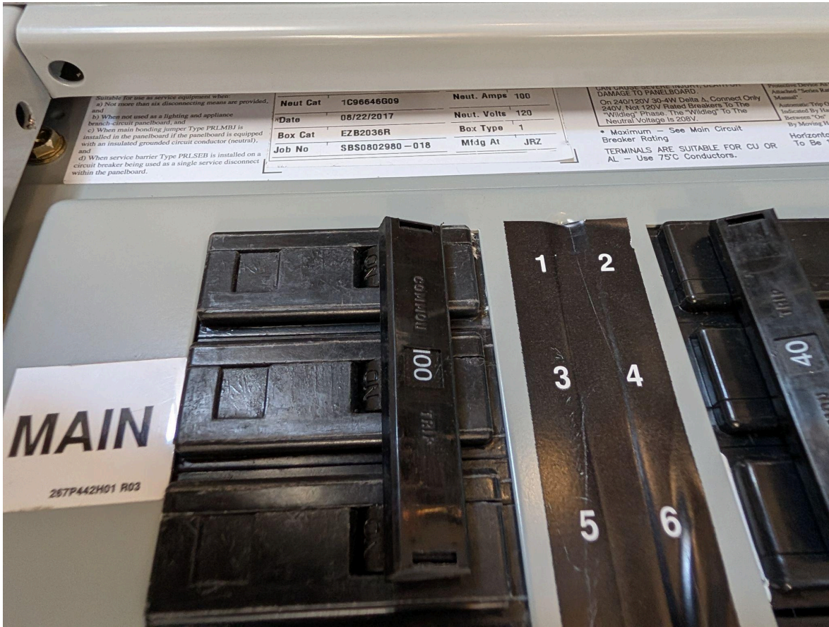
Pump House Panel (picture 1)
