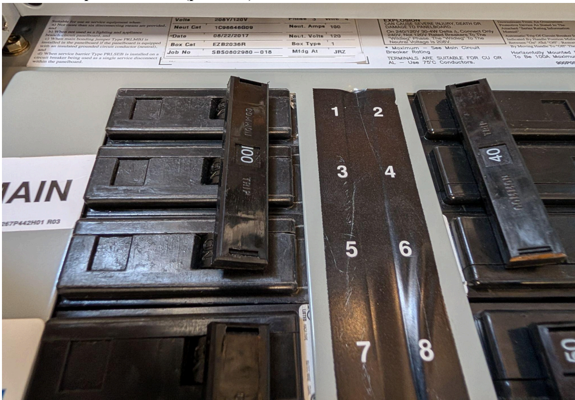
Pump House Panel (picture 2)
