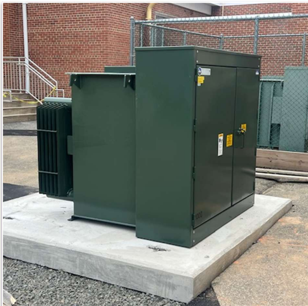
Transformer Placement at CAS
