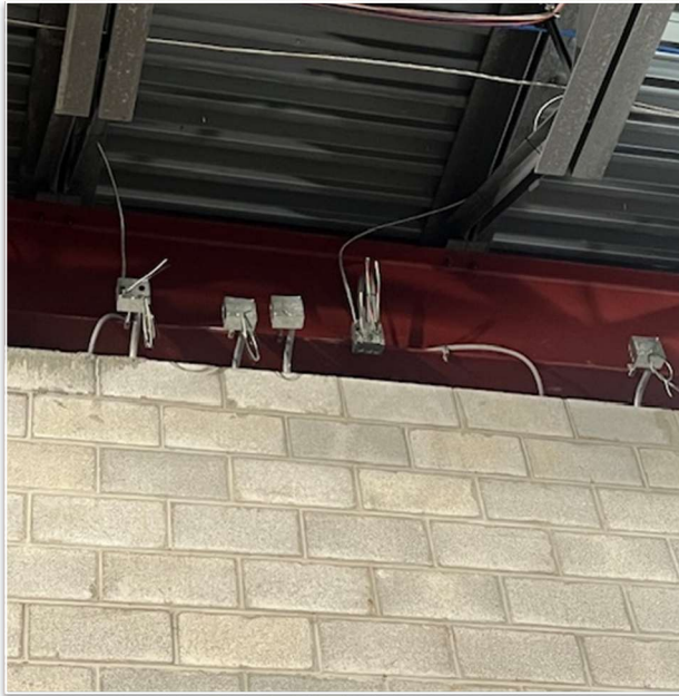
Above Ceiling Electrical at KRS
