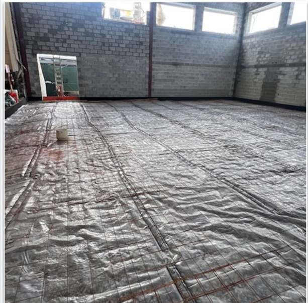
Electrical for Heaters at KRS
