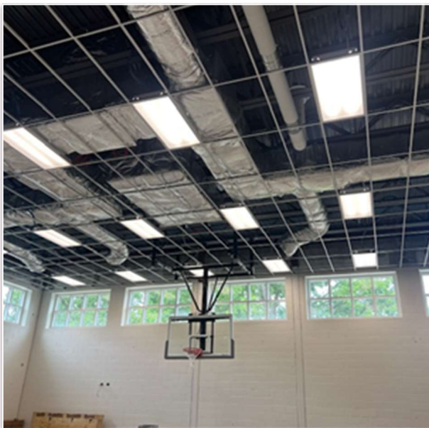
Lights in Ceiling Grid at KRS
