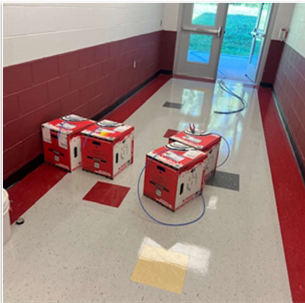
Data/ CAT 6 Lines at CAS
