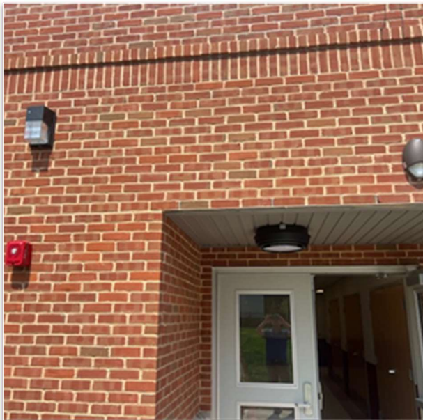
Emergency Lights at CAS
