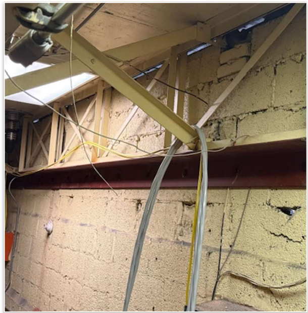
HVAC Room Wall Bracing at KRS
