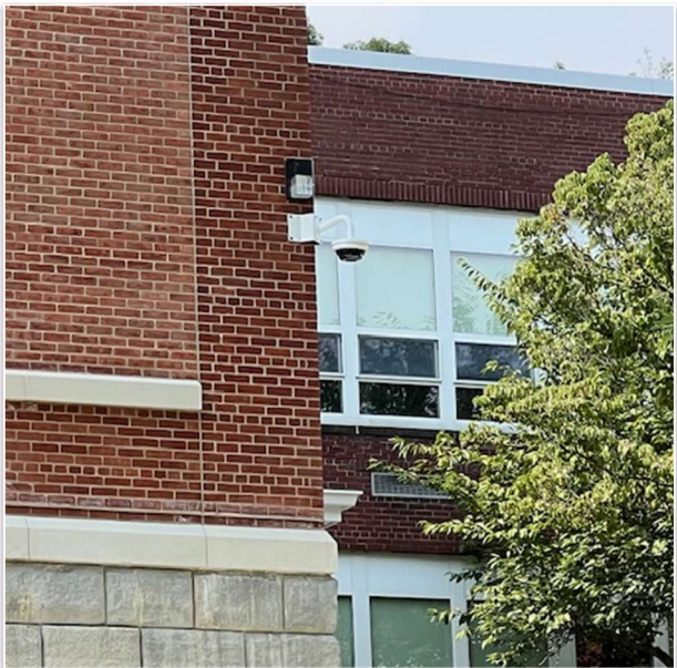
Camera Installation at KRS
