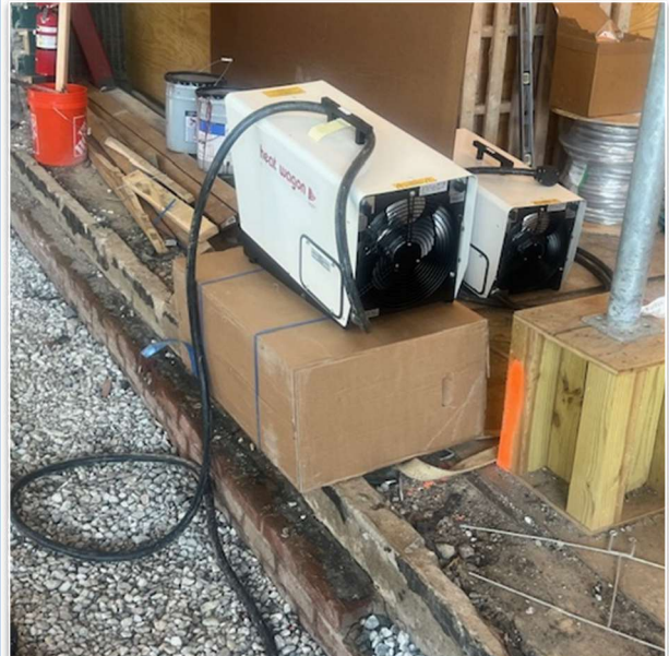
Temporary Heaters at KRS
