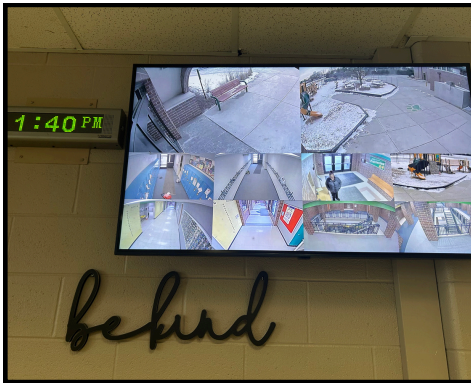
New intercom systems installed at Prairieview and new camera systems with larger monitors at all schools.
