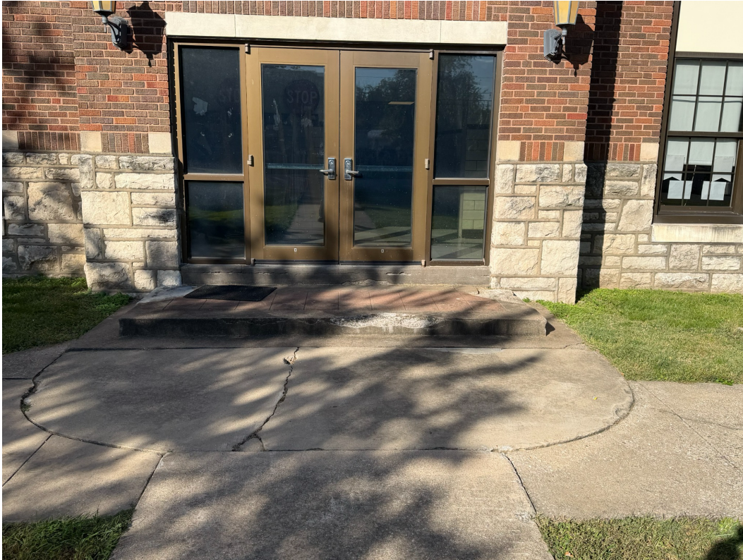
Entryway north of the main entrance - existing concrete section and step proposed for removal/replacement
