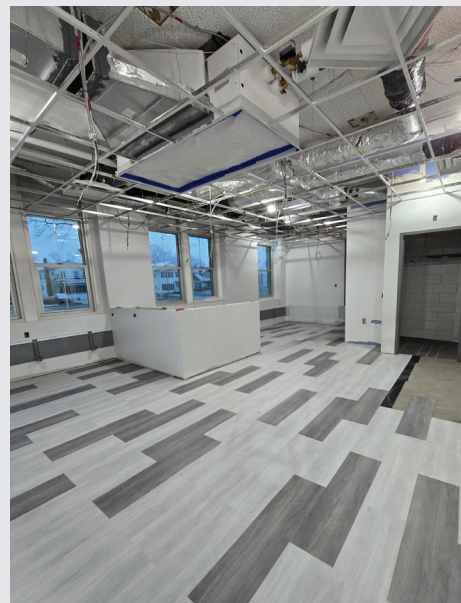
A look at progress on the new nurse's suite at Attica Elementary School, which will be located immediately adjacent to the main building entrance, eliminating the need for parents to enter the school proper when picking up their students.
