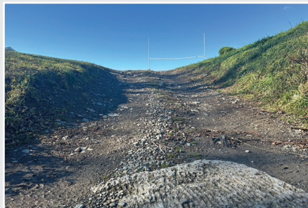
Runoff path used by vehicles, not intended for accessible travel.
