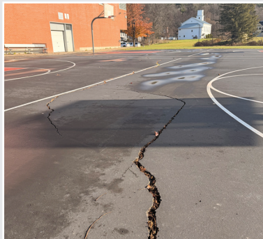
A large crack cuts across the outdoor court, indicating needed repairs.
