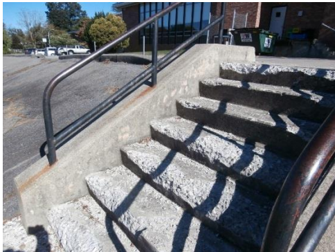
Deteriorated stairs at rear of building
