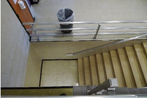
High fall risk at main stair
