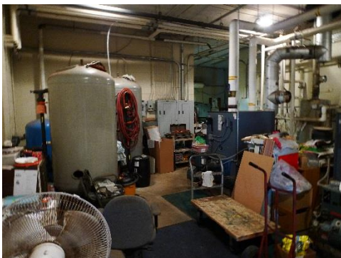
Existing mechanical room
