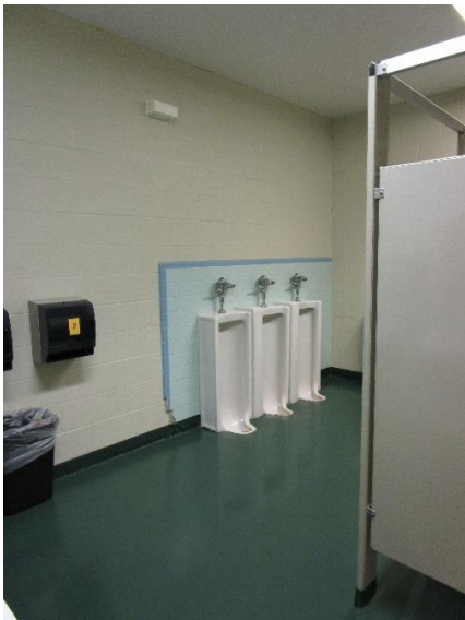
Original plumbing fixtures
