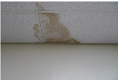
Water damage at upper level ceiling
