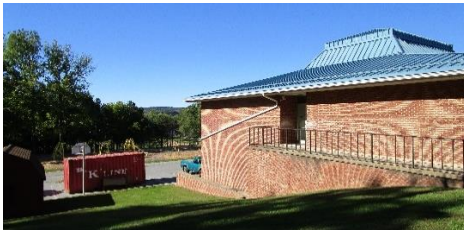
High fall risk at egress path/exterior storage
