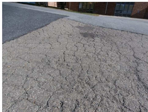
'Alligatoring' and cracked pavement near staff parking (rear of building)
