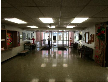
Existing entrance is not secure
