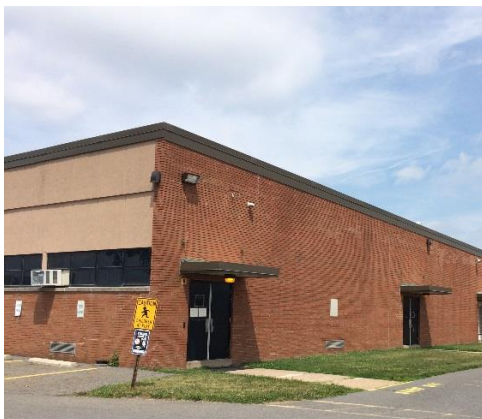
Auxiliary air conditioner at multi-purpose room
