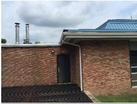
Surface deterioration at roof transitions
