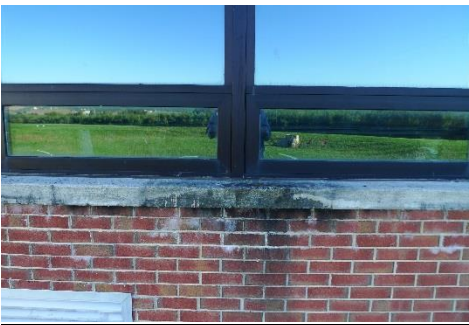
Detail of existing sill deterioration
