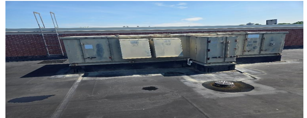
Air handling units on the roof — poor condition, 1999
