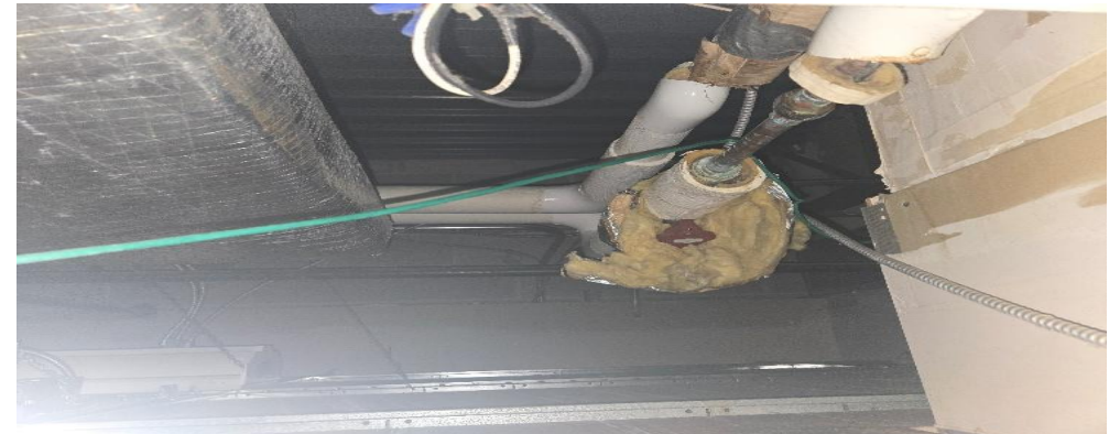
Damaged pipe insulation observed during survey
