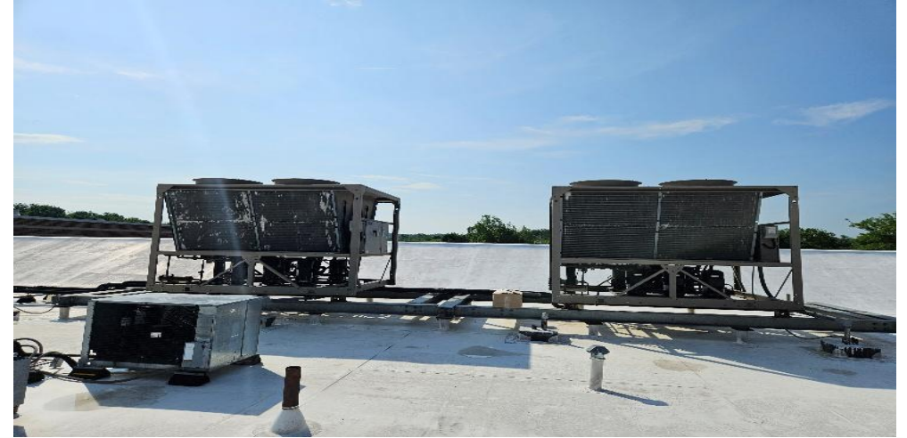
Roof-mounted condensers — poor condition, damaged coils/fins
