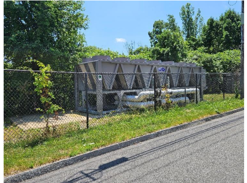
The building's 2022 chiller — an example of what well-maintained, modern equipment looks like
