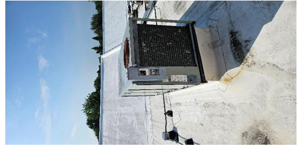
Rooftop unit — 1998, well past 15-year ASHRAE life expectancy
