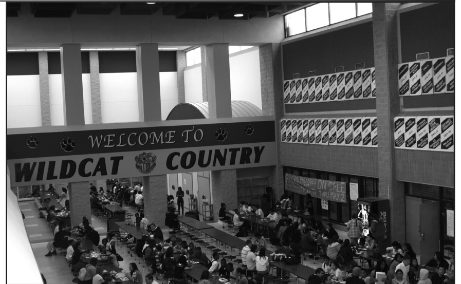
Students enjoy lunch in the commons while the cafeteria is being renovated. The updated theater entrance is in the background.
