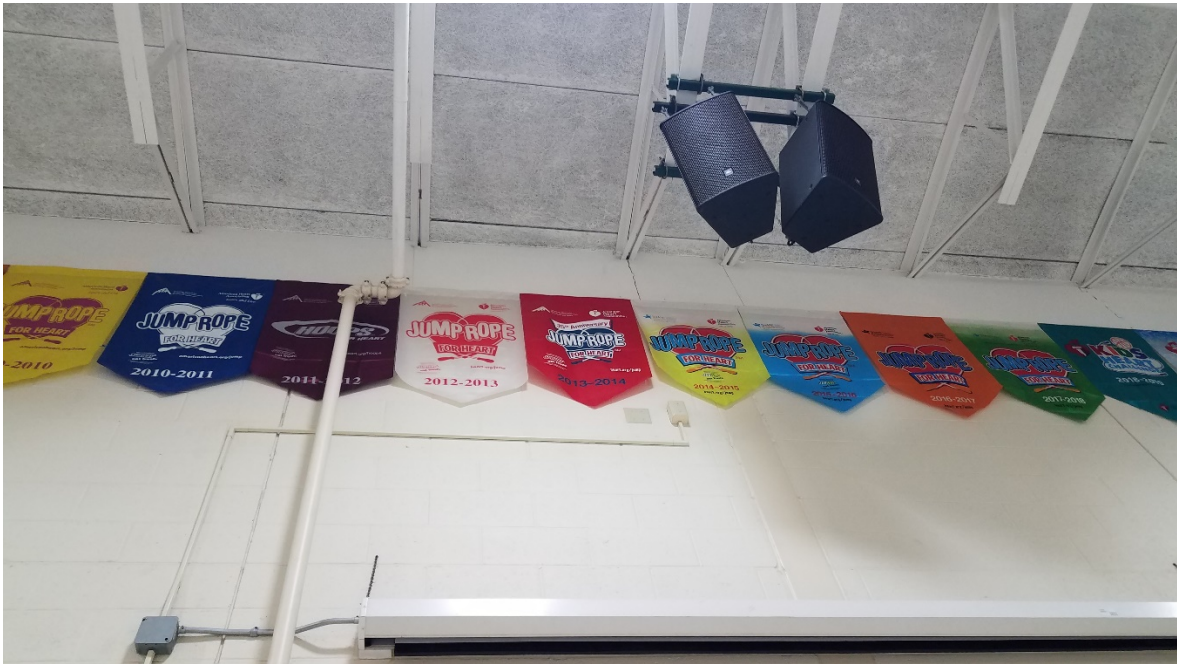
Vertical Cracks at Gymnasium
