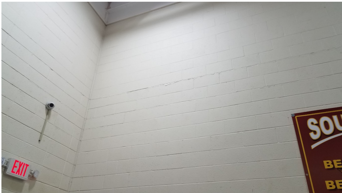
Horizontal Crack at Gymnasium
