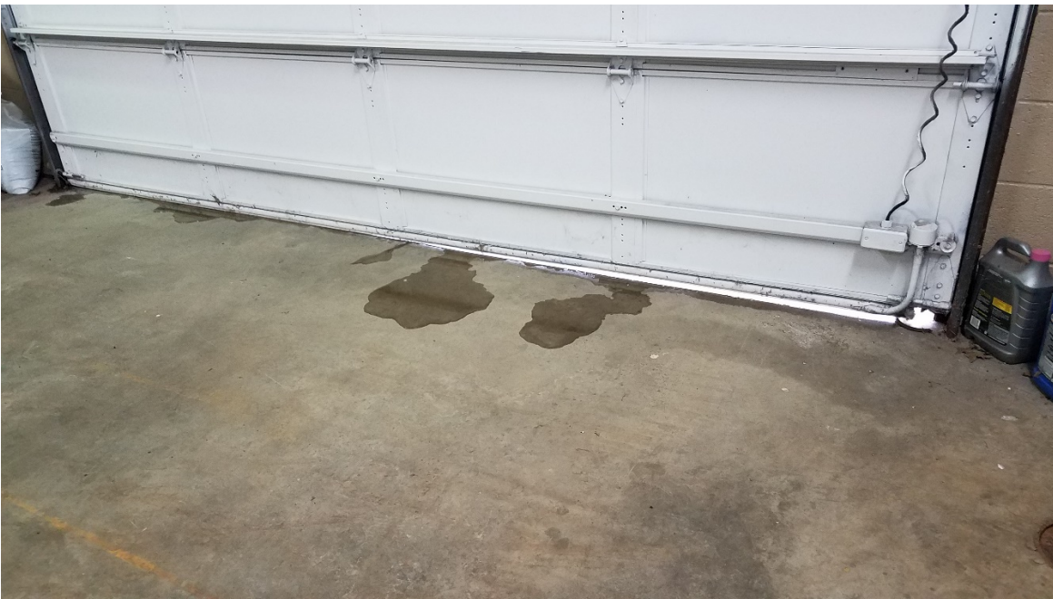
Garage Door Leak During Rain Storm
