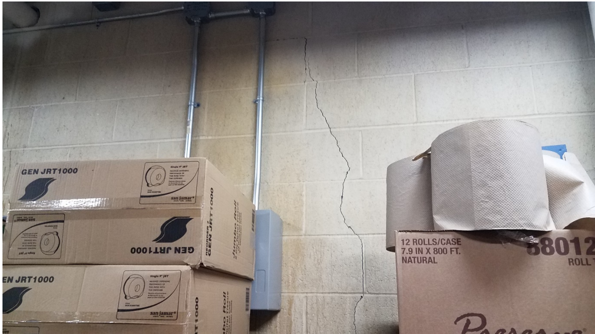
Vertical Crack in Main Electrical Room
