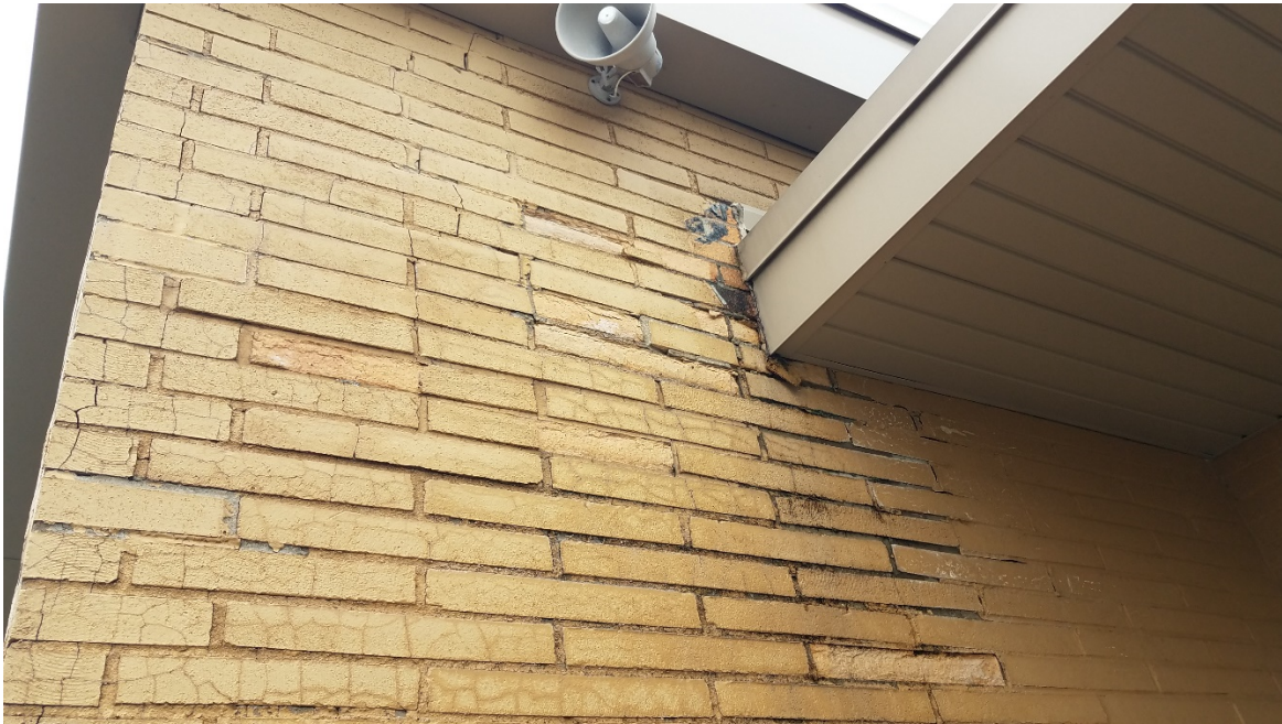
Spalling and Cracking Brick at High School
