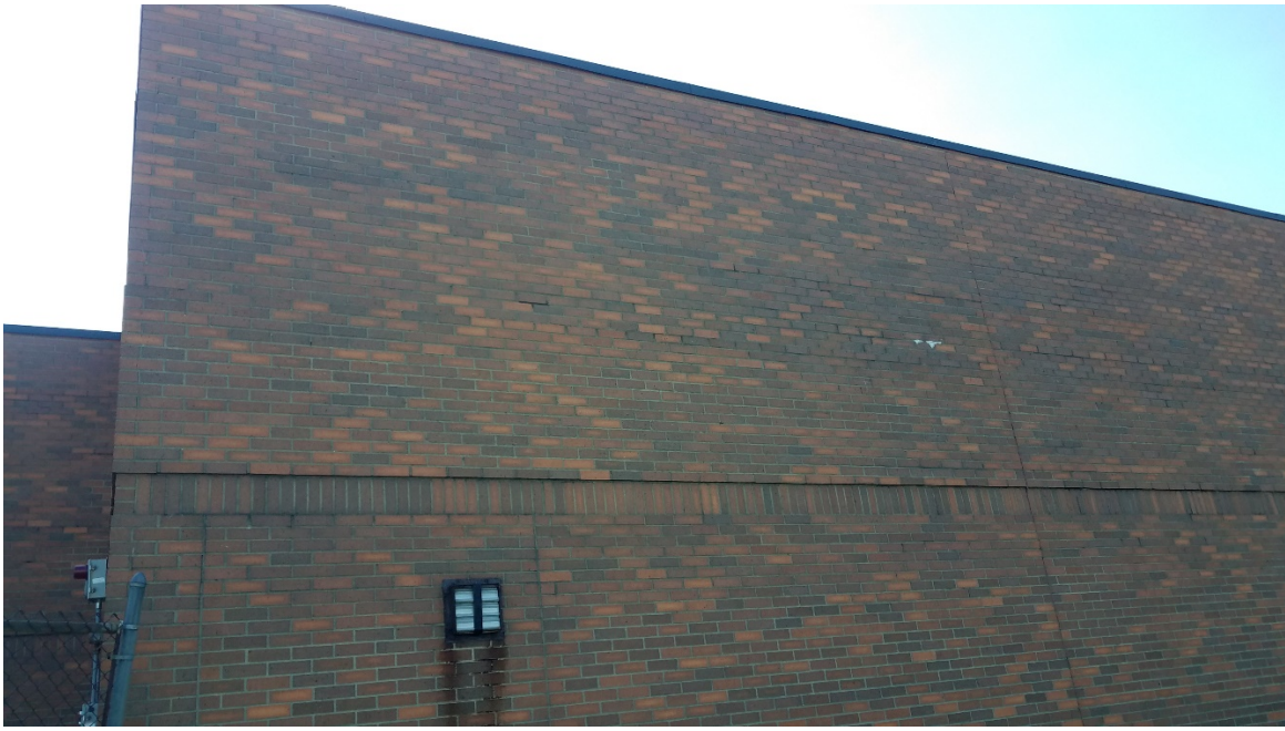
Partial Height Control Joint at Corner – Full Height Control Joint approx. 20ft from Corner
