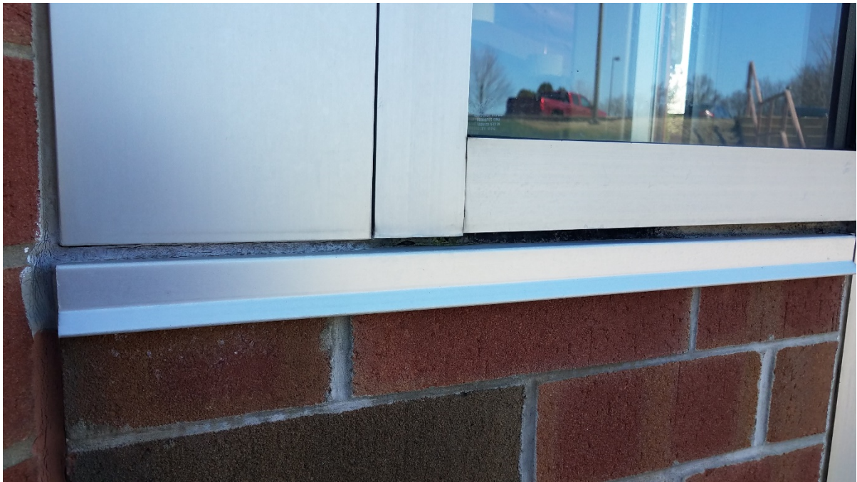
Sealant at Windows
