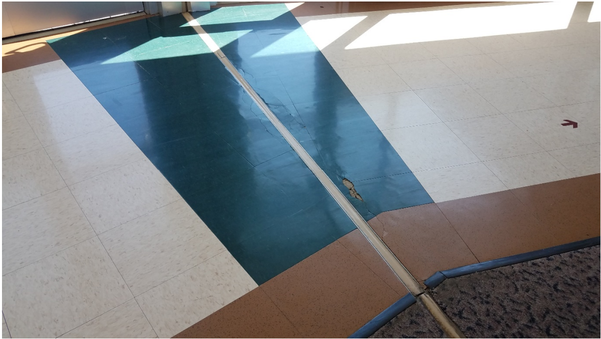
Cracking at Expansion Joint
