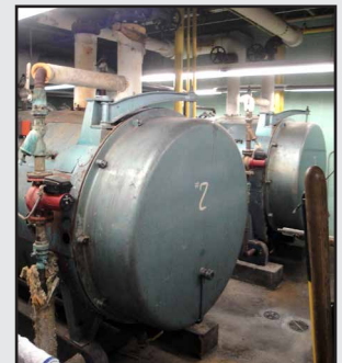
QUEST boiler plant
