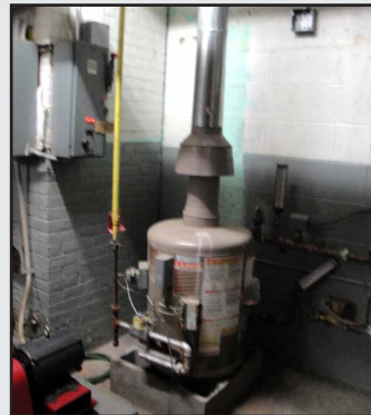
Village water heater
