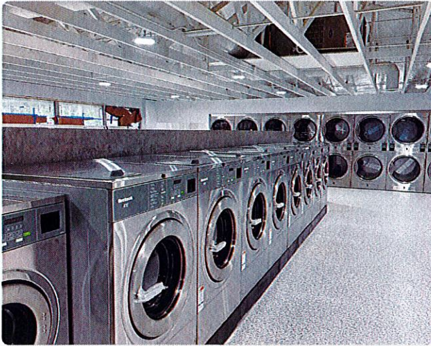
Washer and dryer bank, main floor
