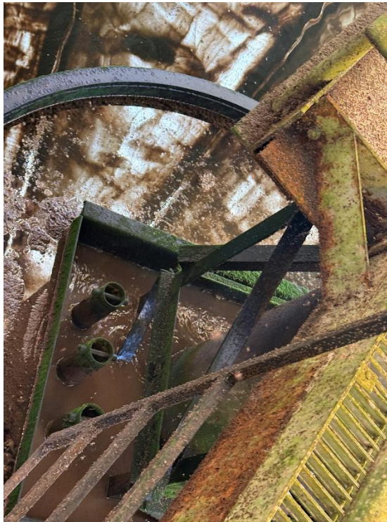
Figure 2: Clarifier Sludge Drawoff Box
