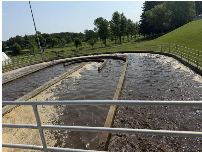
Figure 1 – Existing Oxidation Ditch
