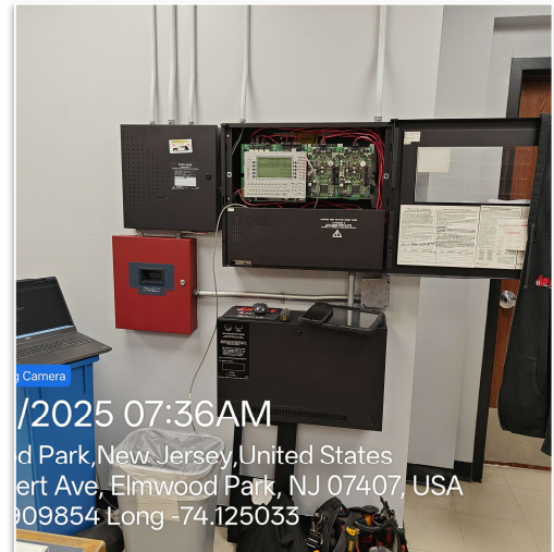
Gilbert- Addition Fire Alarm connected to the Main Panel
