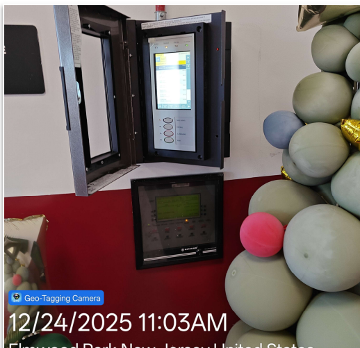
16th-Additon Fire Panel tied into the Main Panel
