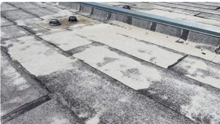
Photo showing granules piled up from field deterioration.
