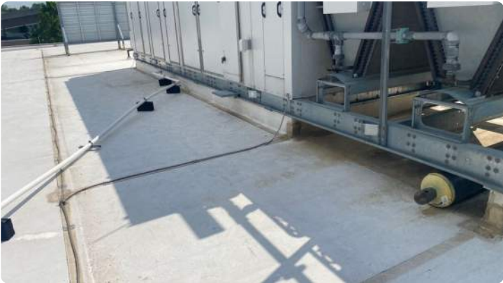
Photo showing condition if the projection flashings.
