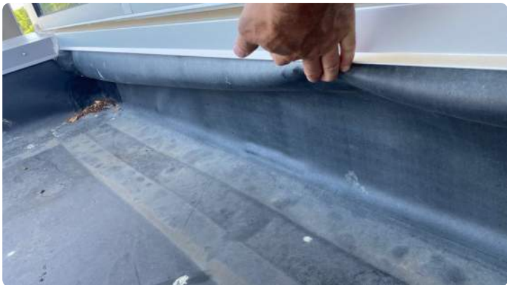
Photo showing loose membrane along perimeter.
