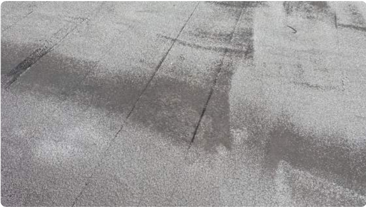
Photo showing scrim showing through deteriorated roof and loose granules piling up from deteriorated roof.
