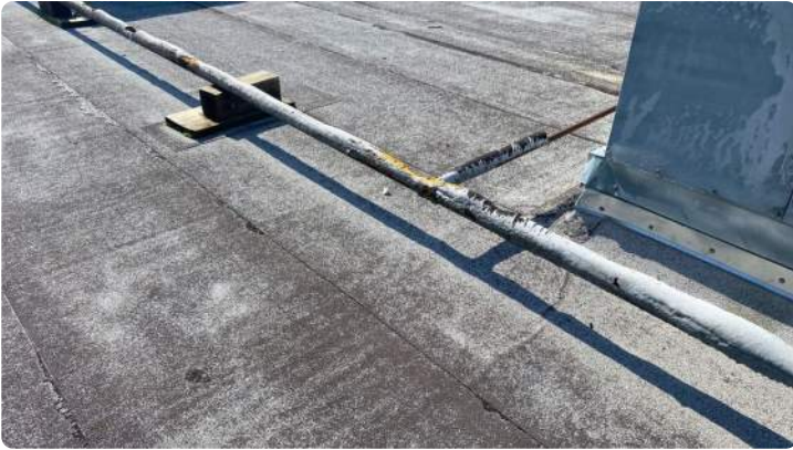
Photo showing deteriorating field.
