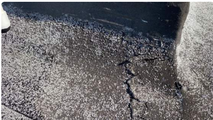
Photo showing skim exposed in cracking projection flashings.
