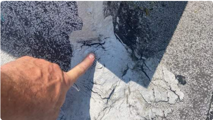
Photo showing crack in the projection flashings.
