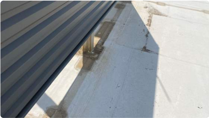
Photo showing condition if the projection flashings.
