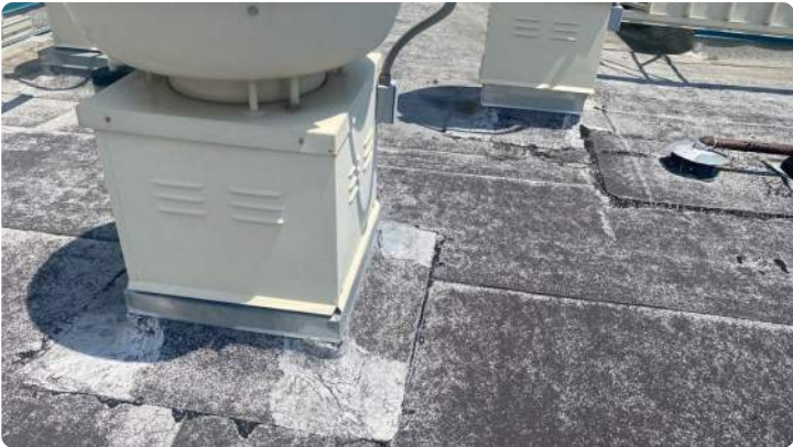
Photo showing condition of the projection flashings and deteriorating field.
