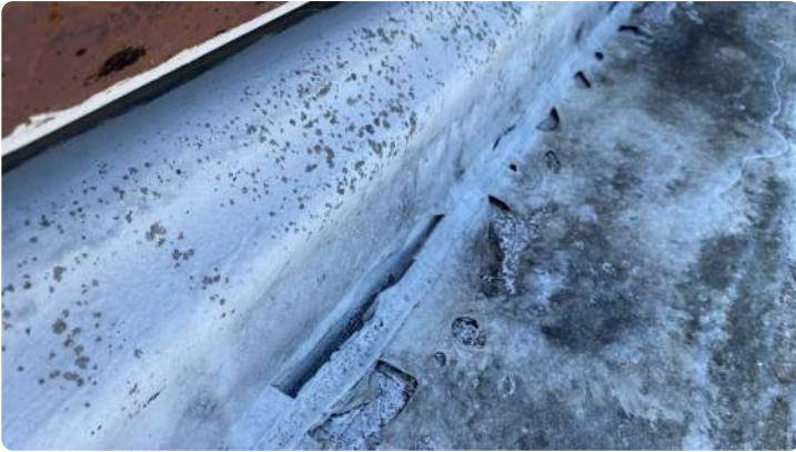
Photo showing coating deteriorating along the perimeter flashings.
