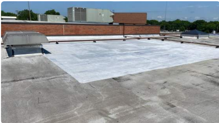
Photo showing area with aluminum coating.
