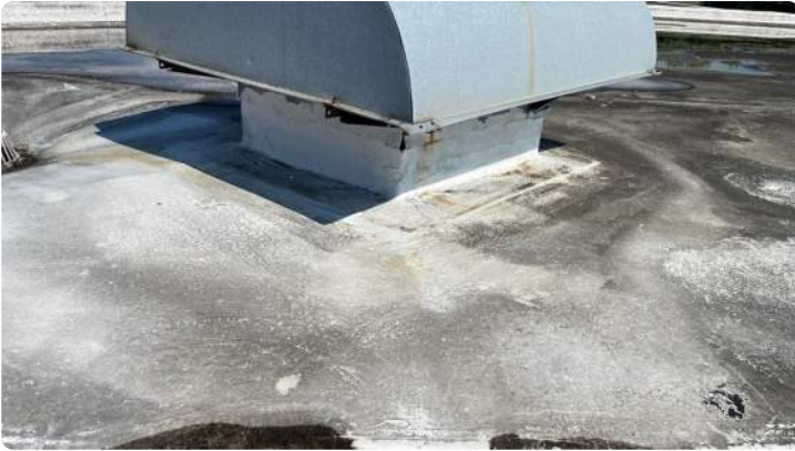
Photo showing condition of the projection flashings.
