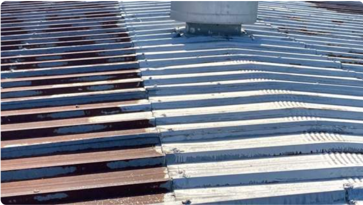
Photo showing deterioration of metal roof.
