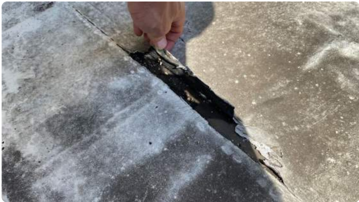
Photo showing coating pulling up at seams.
