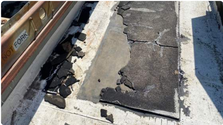
Photo showing walk pads deteriorating.
