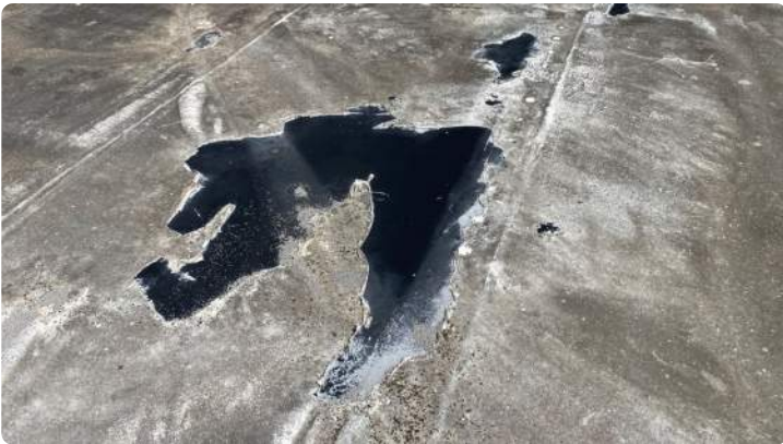
Photo showing deteriorating coating.
