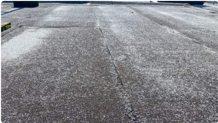
Photo showing deterioration of the field.
