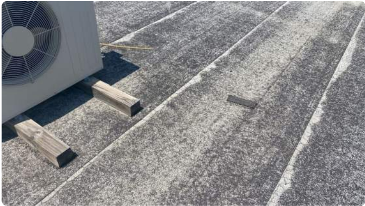
Photo showing area were insulation is soft under field.
