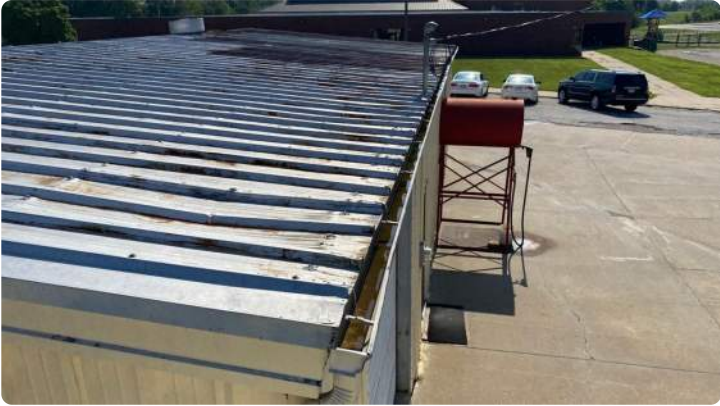
Photo showing condition of the gutter edge.
