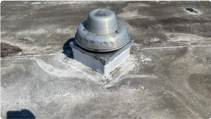
Photo showing condition of the projection flashings.
