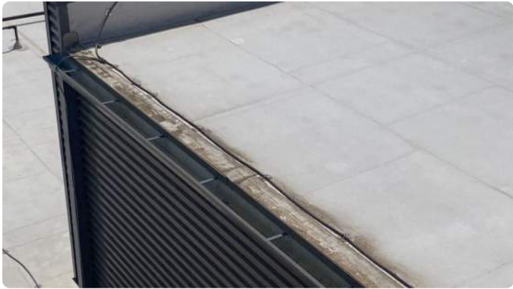
Photo showing condition of the gutter edge.
