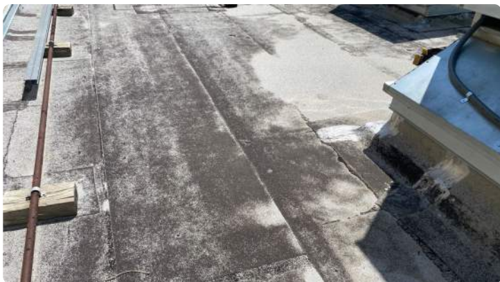
Photo showing deteriorated field.
