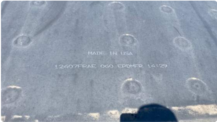
Photo showing manufacturer stamp of EPDM membrane.
