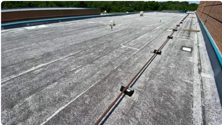
Photo showing deteriorating field.
