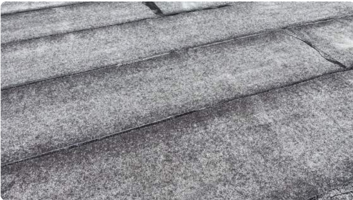
Photo showing scrim visble through deteriorated field.
