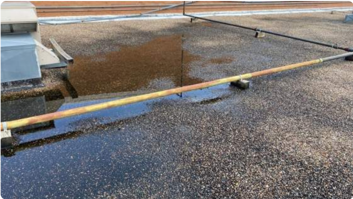
Photo showing additional ponding water.
