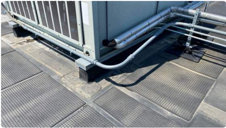
Photo showing condition of the projection flashings.
