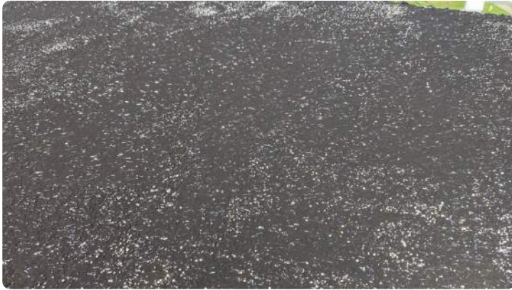
Photo showing deterioration of the coating.
