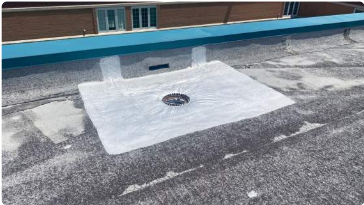
Photo showing drain area coated with aluminum.
