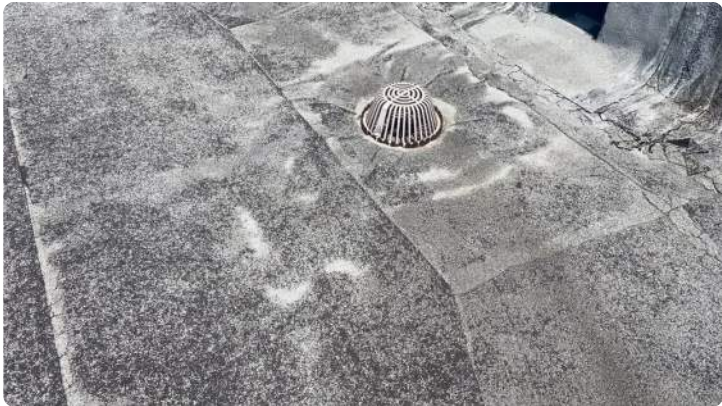
Photo showing deterioration around drain.
