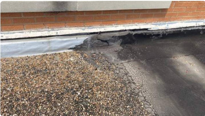
Photo showing perimeter flashing transition coated in deteriorating roofing mastic.
