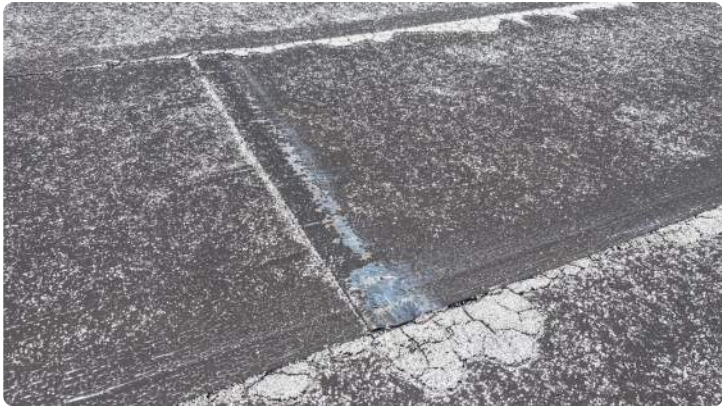
Photo showing skim exposed at seams.
