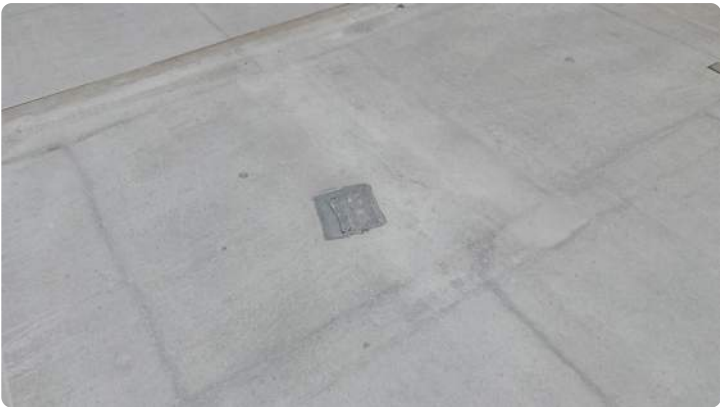
Photo showing additional patch to previous damage.
