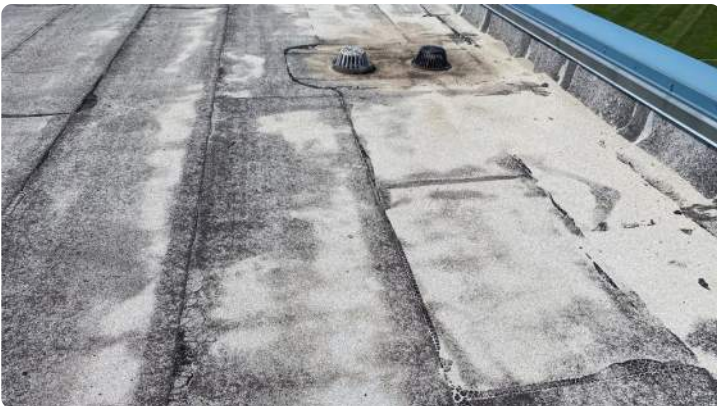
Photo showing granules piled up from deteriorated roof.
