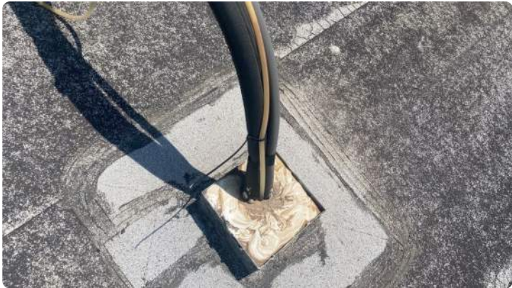
Photo showing condition of pitch pan.
