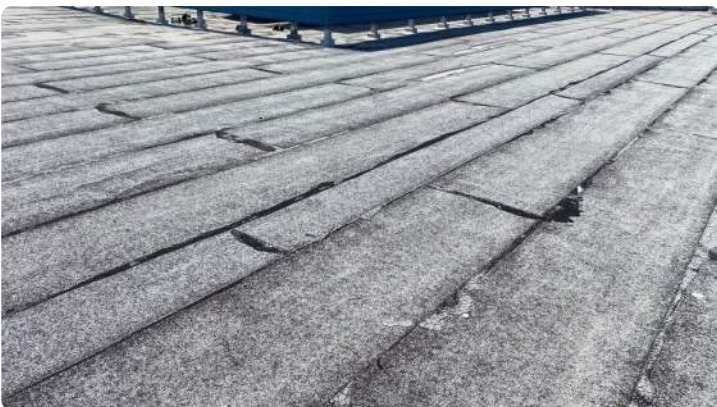
Photo showing deterioration of field.
