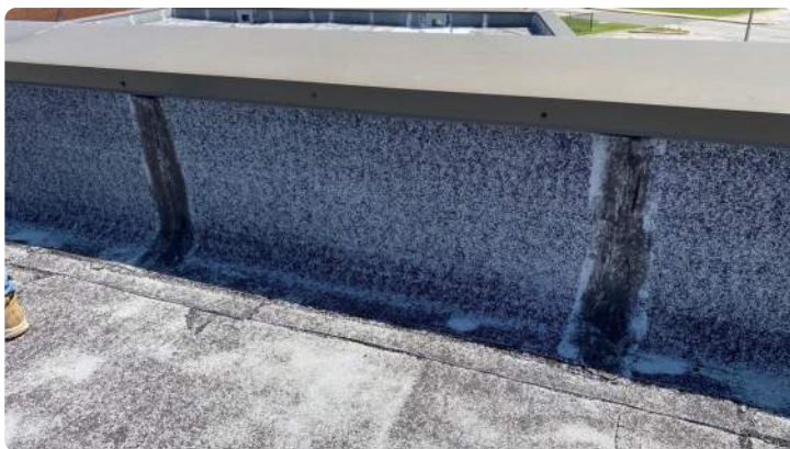
Photo showing condition of the deteriorating perimeter flashings.
