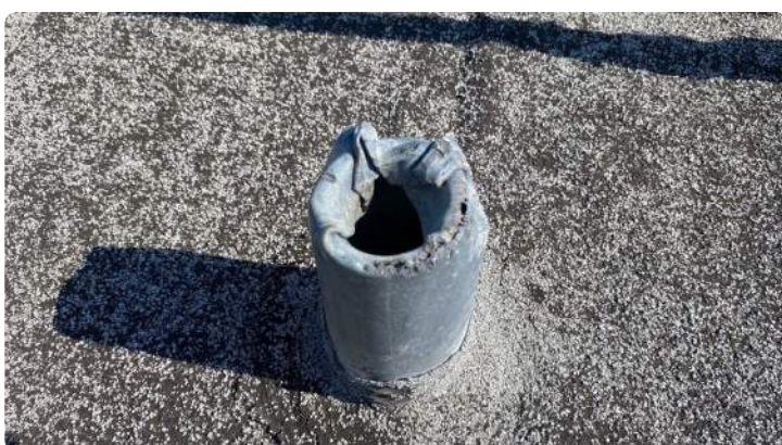
Photo showing cracks in lead covered vent stack. Re-paired as part of the maintenance agreement.
