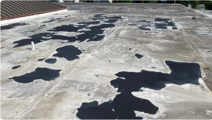
Photo showing deteriorating coating.
