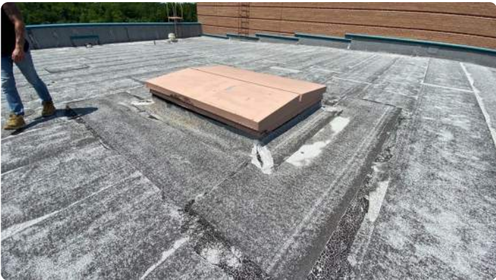
Photo showing condition of the projection flashings.
