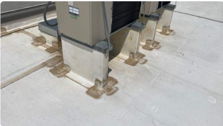
Photo showing condition of the projection flashings.
