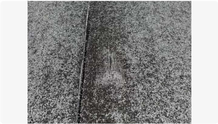
Photo showing exposed scrim in field.
