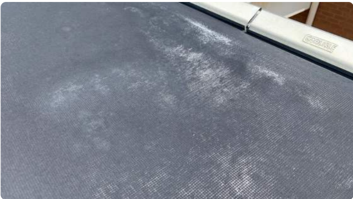
Photo showing skrum showing through deteriorated roof membrane.
