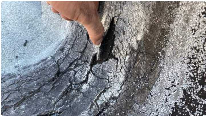
Photo showing additional hole in the perimeter flashings.
