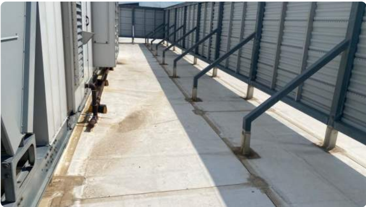
Photo showing condition if the projection flashings.
