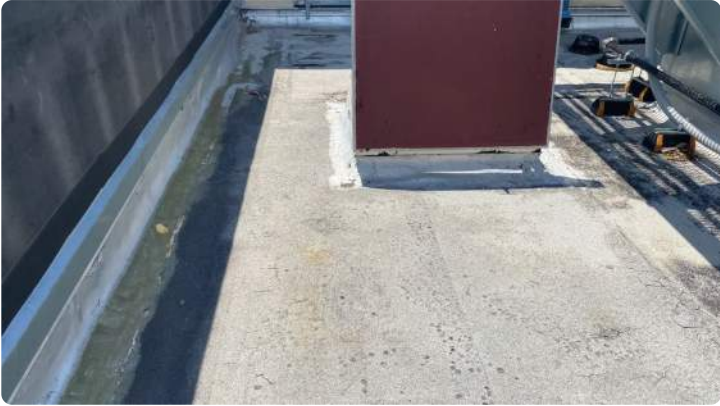
Photo showing condition of area surrounding hatch.
