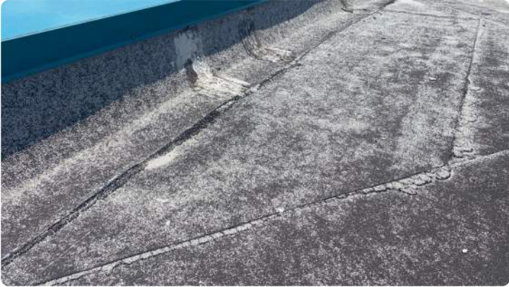
Photo showing deteriorated field.
