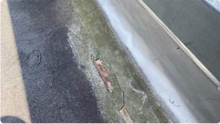
Photo showing coating cracking.
