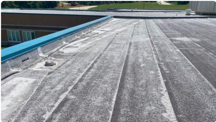
Photo showing additional deterioration.
