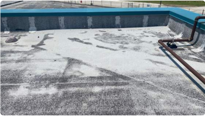
Photo showing granules piled up from deterioration.
