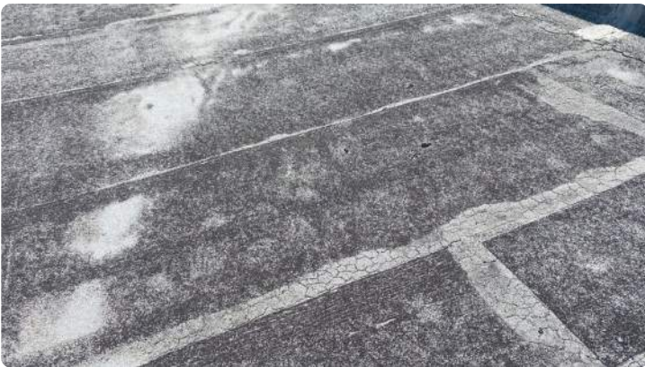
Photo showing deterioration of the field.
