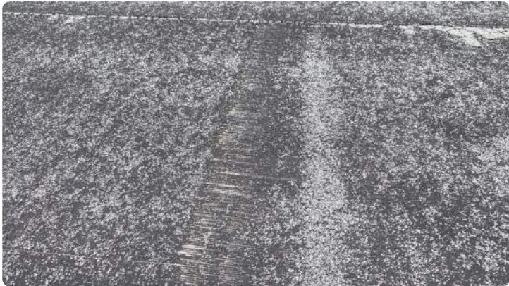
Photo showing skim visible through deteriorating field.
