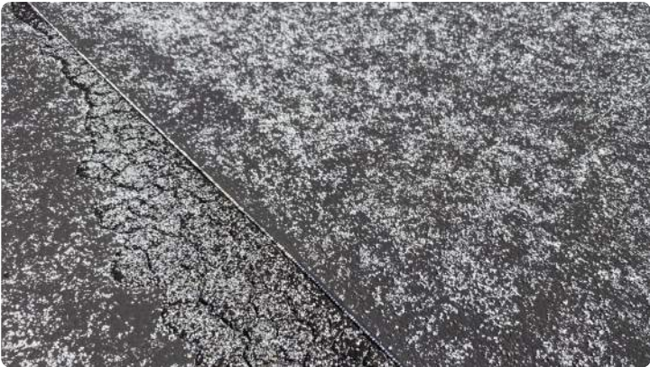
Photo showing skrim showing through deteriorated roof at seams.
