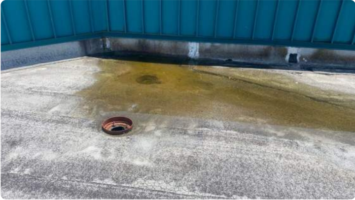
Photo showing drain clogged with trash. Cleared as part of the maintenance agreement.
