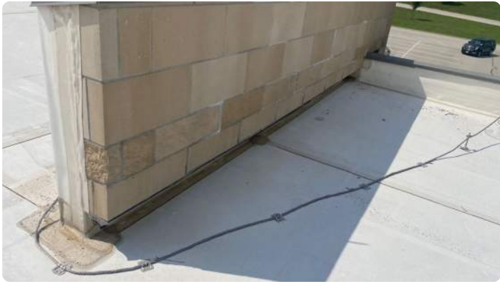
Photo showing condition of perimeter flashings.
