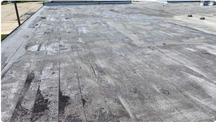
Photo showing scrim showing through deteriorated roof.
