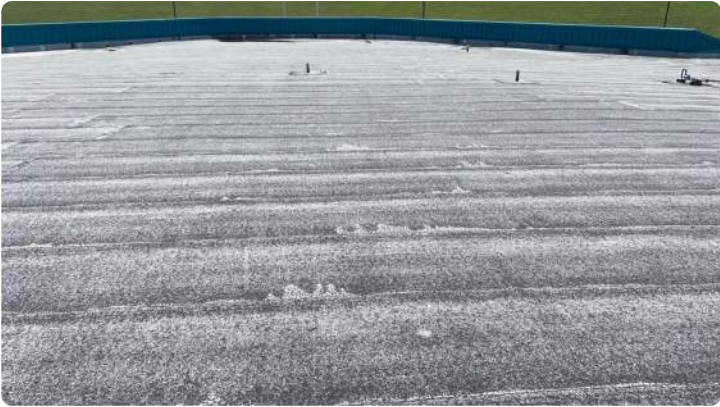
Photo showing field deterioration.
