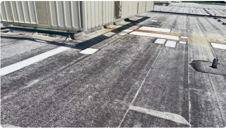
Photo showing previous coating repairs made to field around unit.
