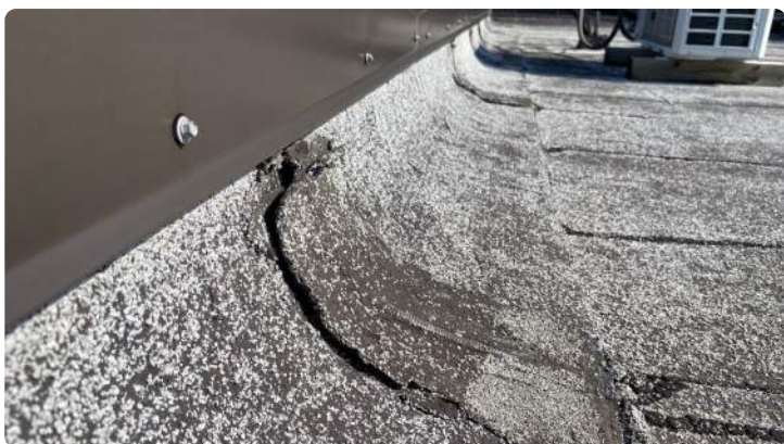
Photo showing crack in the perimeter flashings.
