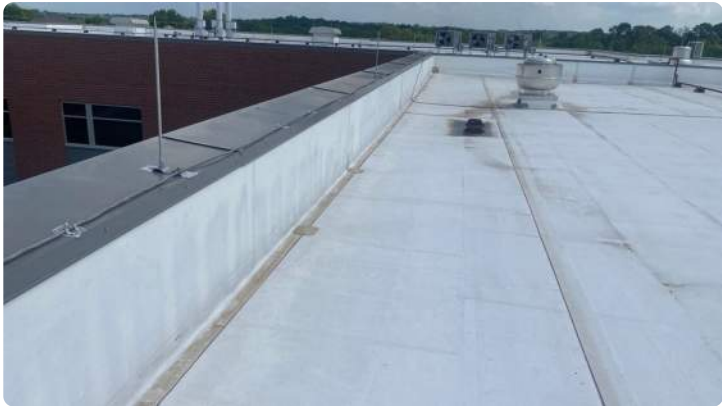
Photo showing condition of perimeter flashings.
