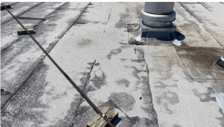
Photos showing granules piled up from deteriorating field.
