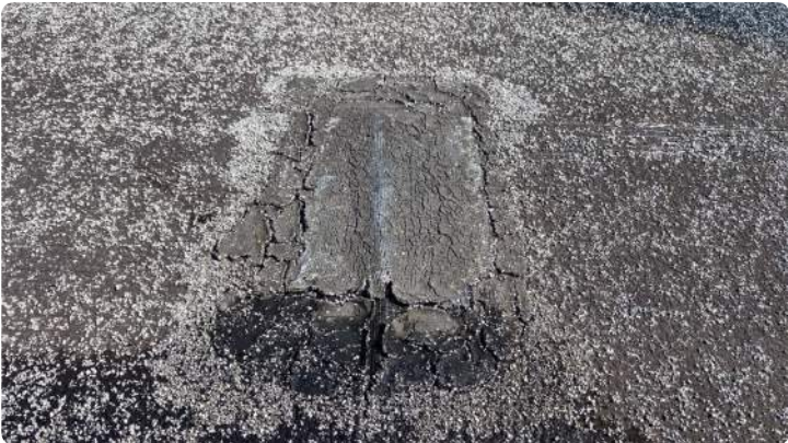
Photo showing deteriorating existing patch.
