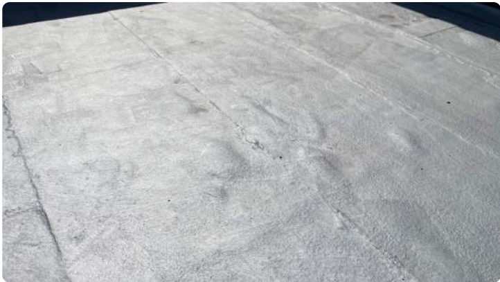
Photo showing minor blistering in field.
