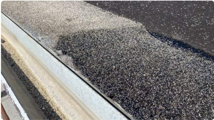
Photo showing deterioration of the coating.
