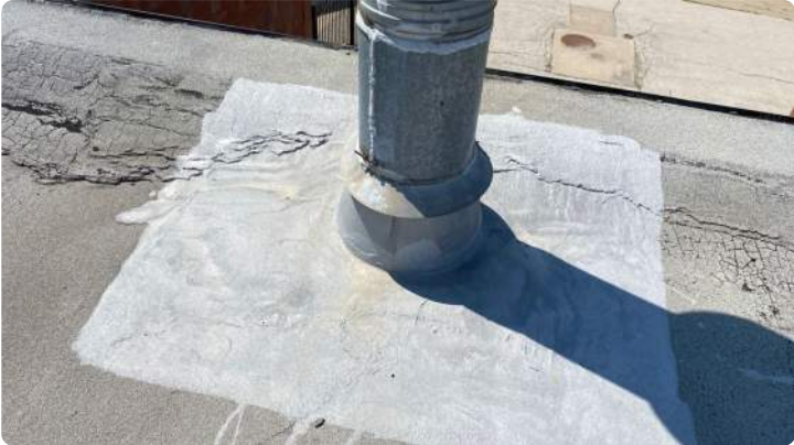
Photo showing additional area with aluminum coating.
