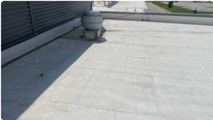
Photo showing condition of perimeter flashings.
