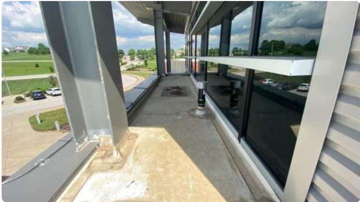
Photo showing condition of perimeter flashings.
