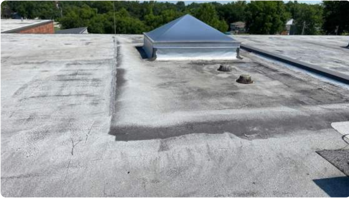
Photo showing condition of small expansion joint section.
