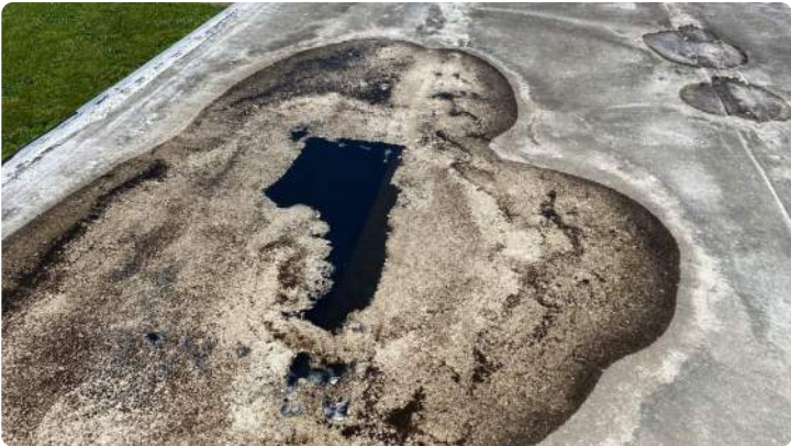
Photo showing deteriorating coating.
