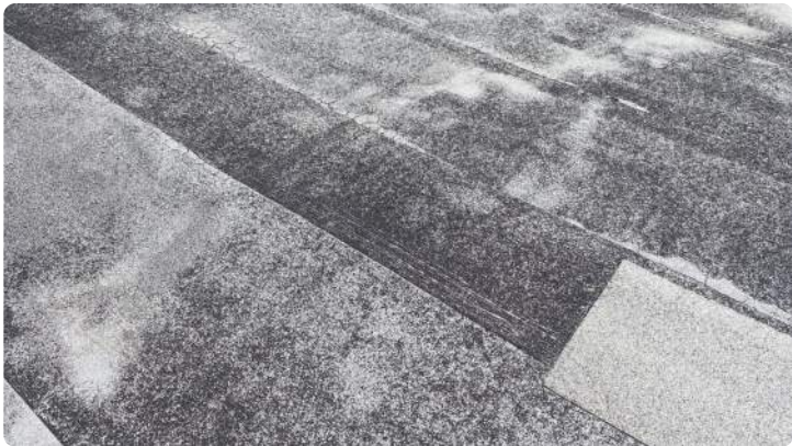
Photo showing additional skim exposed in deteriorated field.
