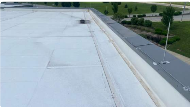
Additional photo showing condition of perimeter flashings.
