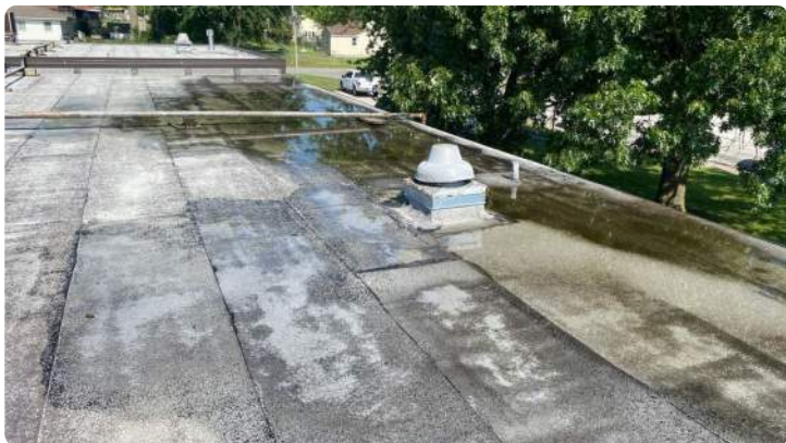
Photo showing additional ponding water.
