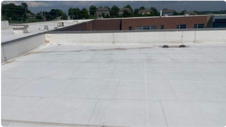
Photo showing condition of perimeter flashings.
