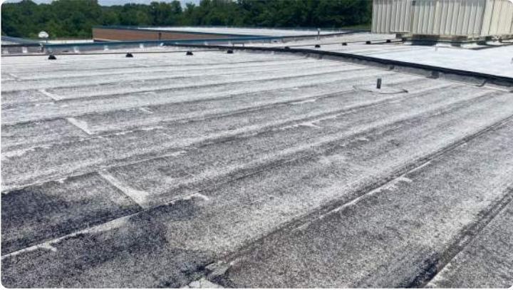
Photo showing deterioration in field.
