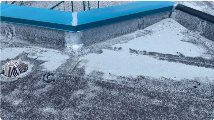
Photo showing granules piled up from deterioration.
