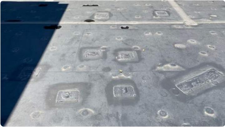
Photo showing multiple patches from previous holes.
