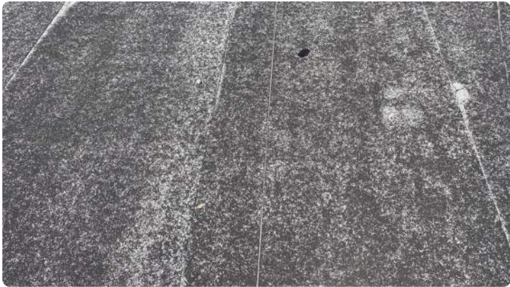
Photo showing scrim visible through deteriorating field.
