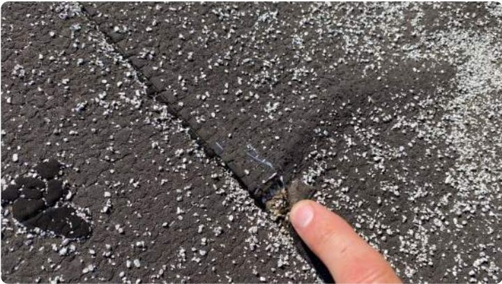
Photo showing hole in the field membrane. Repaired as part of the maintenance agreement.
