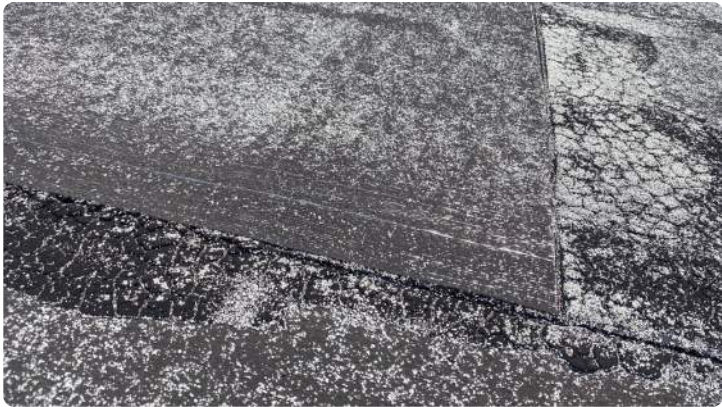
Photo showing deterioration in field.
