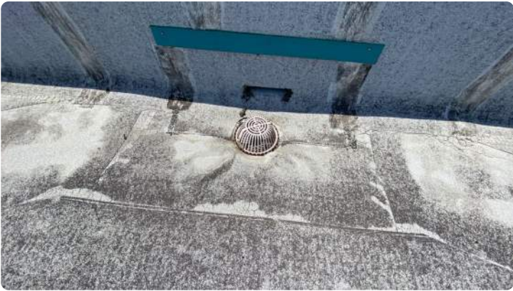
Photo showing granules and wrinkles around drain.
