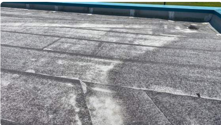
Photo showing loose granules and field deterioration.
