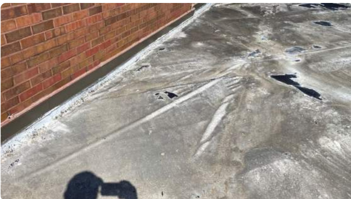
Photo showing deteriorating coating and loose membrane.
