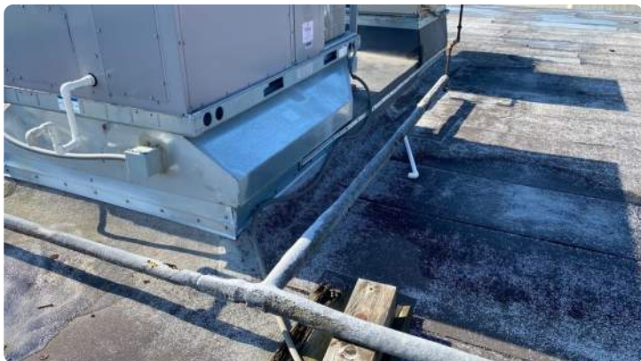
Photo showing condition of the projection flashings.
