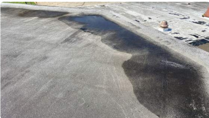
Photo showing minor ponding water along perimeter.
