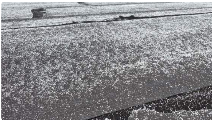
Photo showing scrim showing through deteriorated roof.
