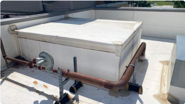
Photo showing condition of the projection flashings.
