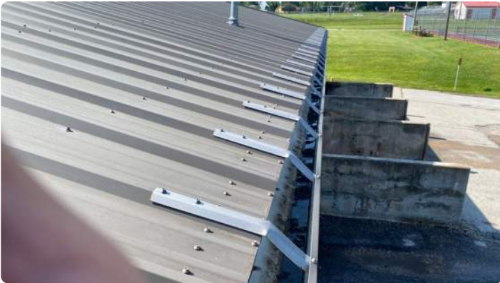
Photo showing condition of the gutter edge.
