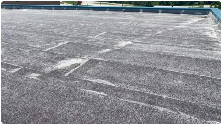
Photo showing deterioration of the field.
