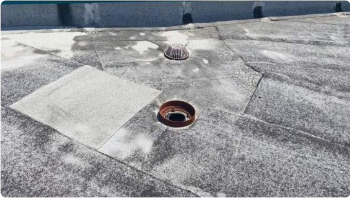
Photo showing blisters around drains.
