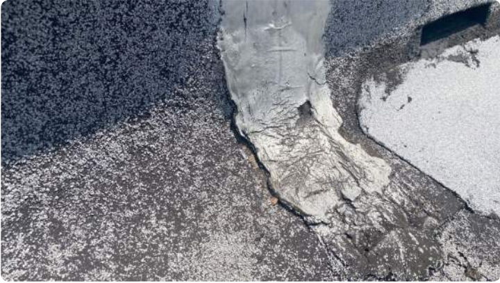
Photo showing deteriorating details.
