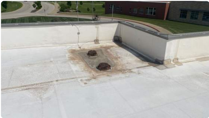
Photo showing condition of perimeter flashings.
