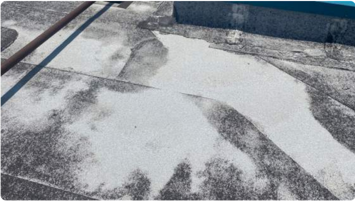
Photo showing granules piled up from deterioration.
