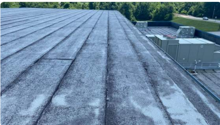
Photo showing additional deterioration of the field.
