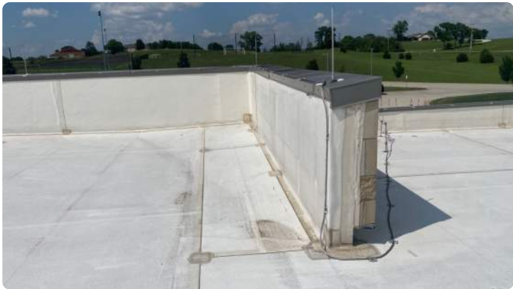
Photo showing condition of perimeter flashings.
