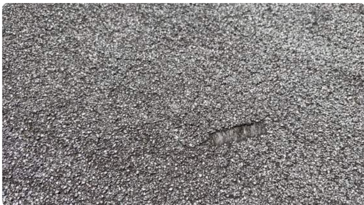
Photo showing skim showing through deteriorated roof and splitting.
