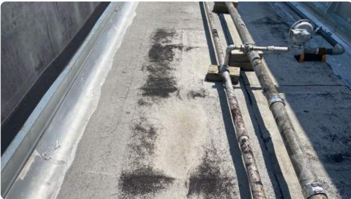
Photo showing more field deterioration.
