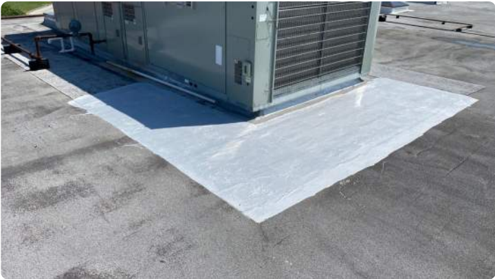
Photo showing aluminum coated area around projection.
