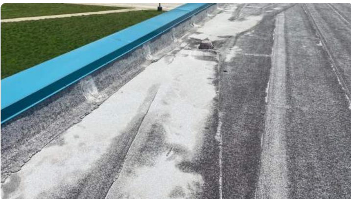
Photo showing granules piled up from deterioration.
