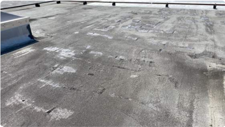
Photo showing scrim showing through deteriorated roof.
