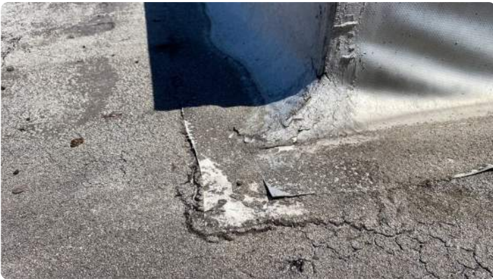
Photo showing deteriorating projection flashings.
