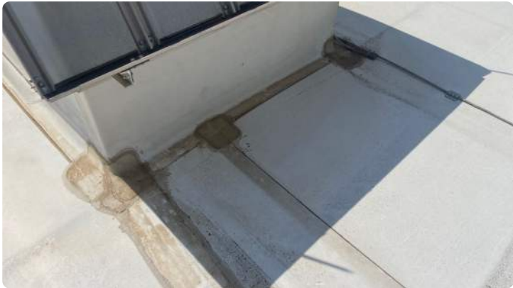
Photo showing condition of perimeter flashings.
