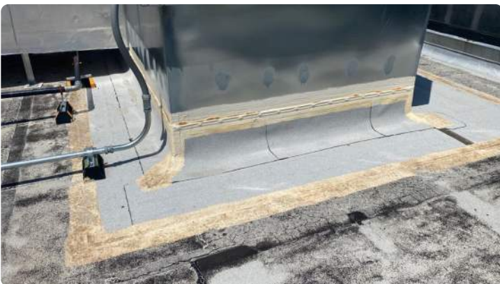
Photo showing condition of the projection flashings.
