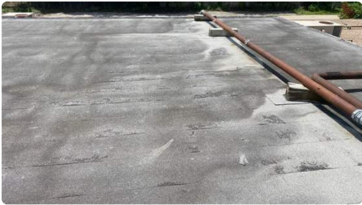
Photo showing skim showing through deteriorated roof.
