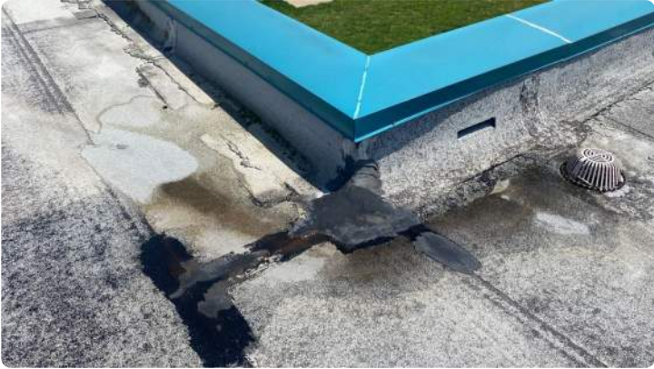
Photo showing corner with multiple openings that was repaired.
