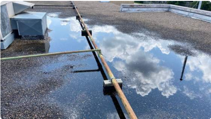
Photo showing ponding water.
