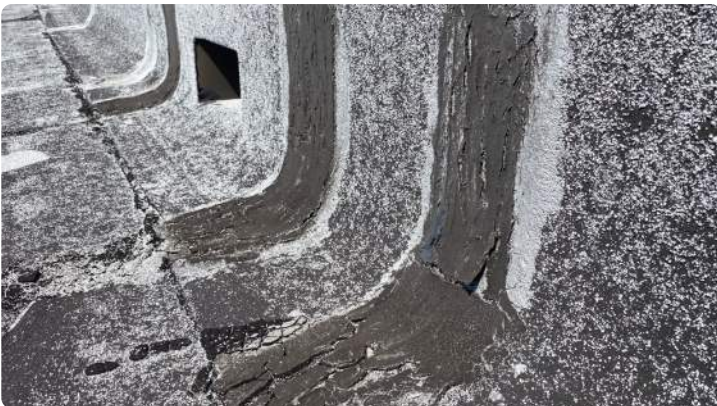
Photo showing perimeter flashing seam reinforcement beginning to deteriorate.
