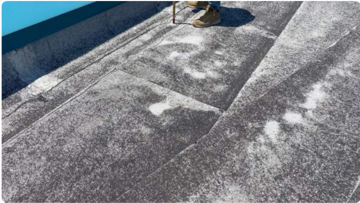
Photo showing deterioration of the field.
