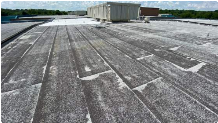
Photo showing deteriorated field.
