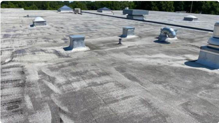
Photo showing skim showing through deteriorated roof.
