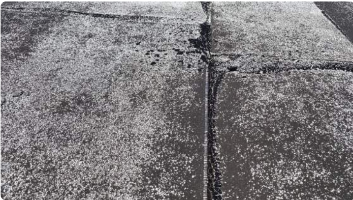
Photo showing skim coming through in the field due to deterioration.
