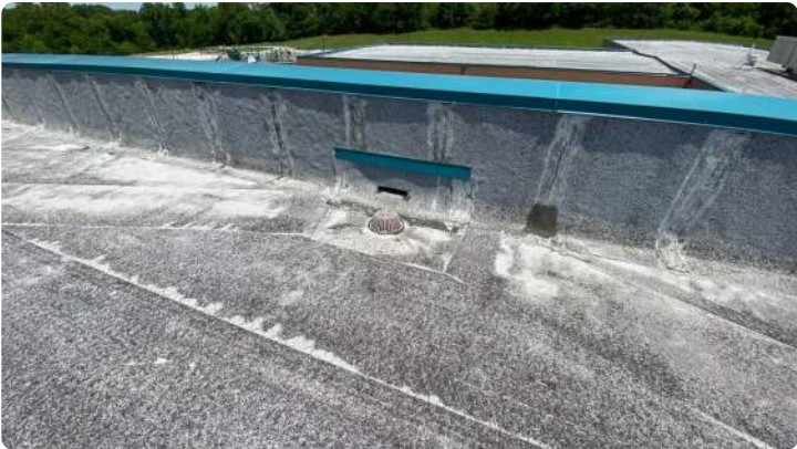
Photo showing condition of the drain.
