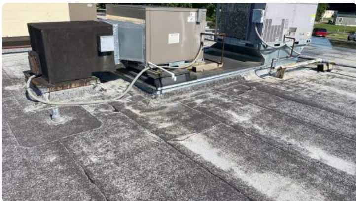
Photo showing deterioration of the field around the units.
