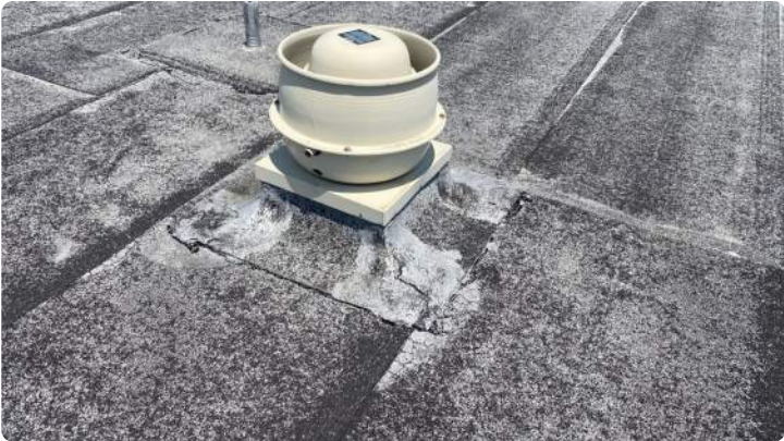
Photo showing condition of projection flashing.
