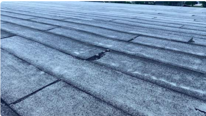
Photo showing deterioration of the field.
