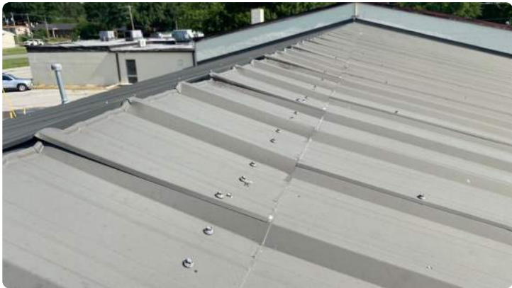
Photo showing fasteners beginning to back out.
