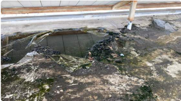
Photo showing coating deteriorating under awning.
