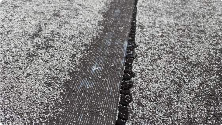
Photo showing skim showing through deteriorated roof.
