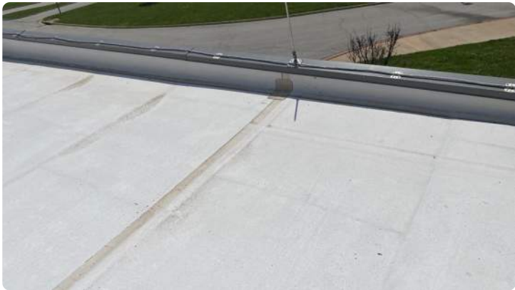
Photo showing condition of perimeter flashings.
