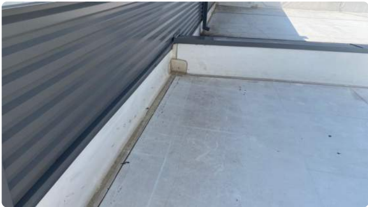
Photo showing condition of perimeter flashings.
