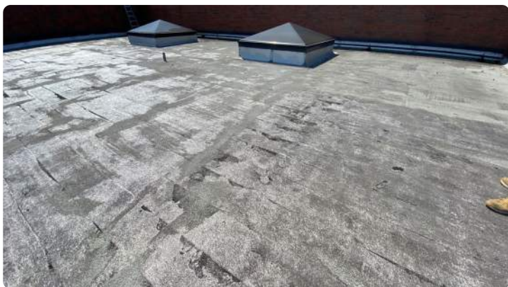
Photo showing scrim showing throughout deteriorated roof.
