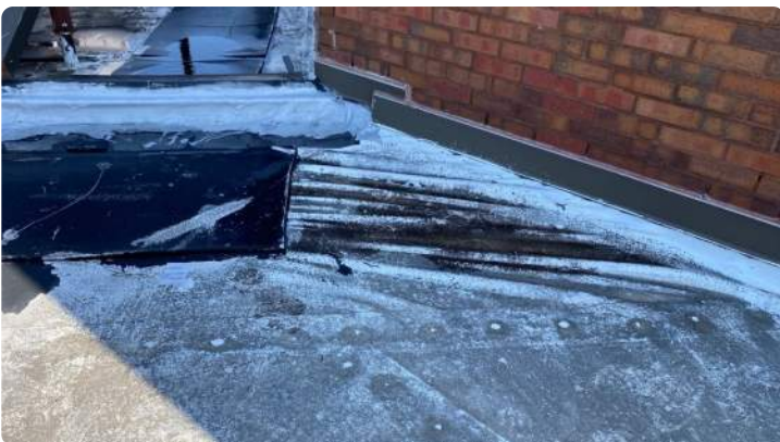
Photo showing coating deteriorating and loose membrane.
