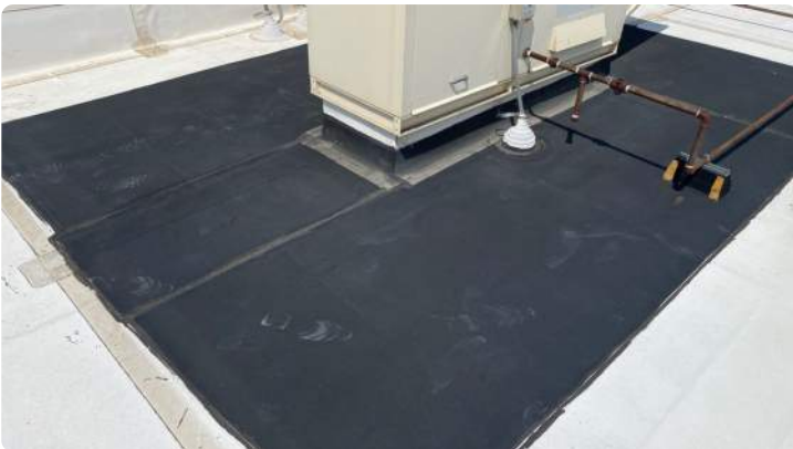
Photo showing condition if the projection flashings with layer of EPDM around unit.
