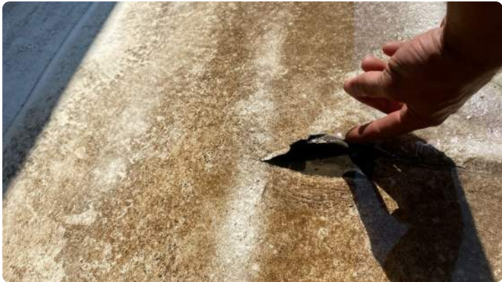
Photo showing coating pulling up.
