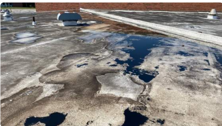
Photo showing deteriorating coating.
