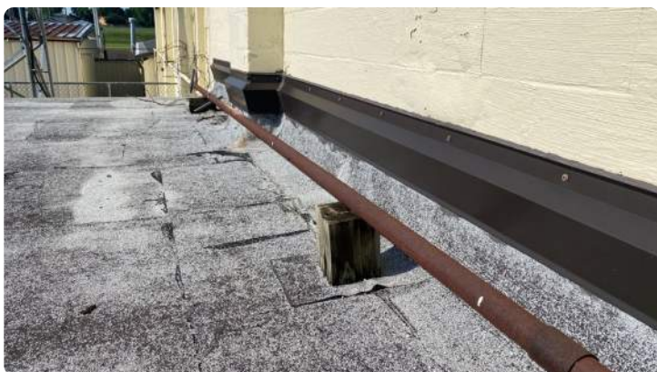
Photo showing blistering in the perimeter flashings.
