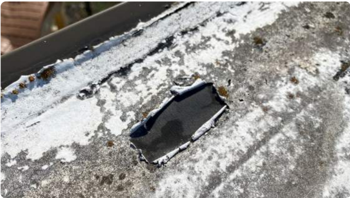
Photo showing deteriorating coating.
