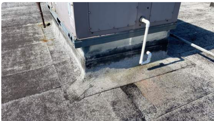
Photo showing deterioration under unit condensation line.
