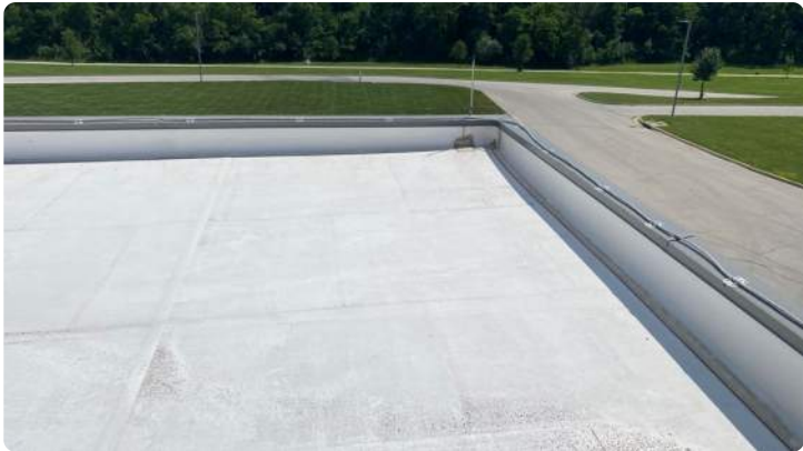
Photo showing condition of perimeter flashings.
