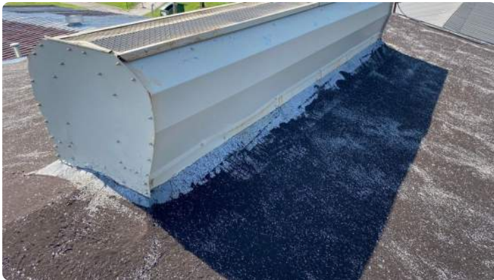
Photo showing condition of the projection flashings.
