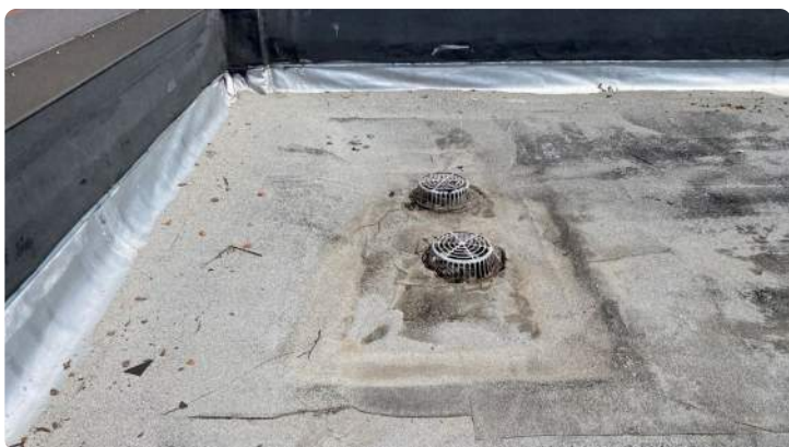
Photo showing granules from deteriorating roof piling up around drain.
