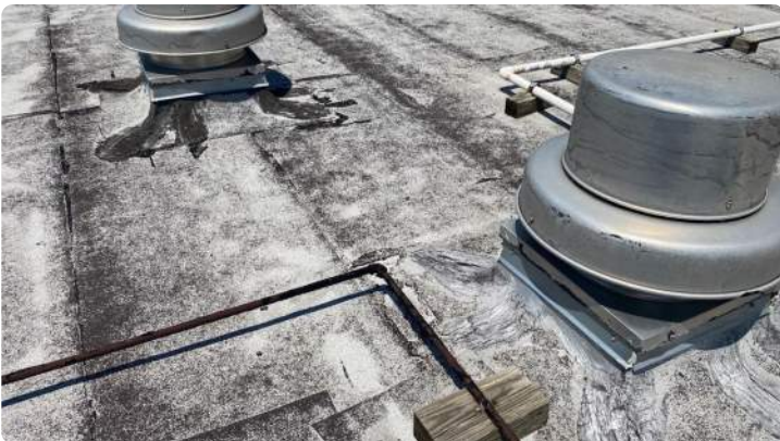
Photo showing condition of the projection flashings and deterioration of the field.
