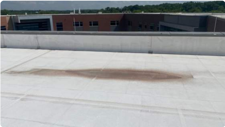
Photo showing minor ponding water.
