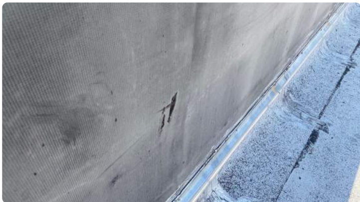
Photo showing deterioration in the perimeter flashings.
