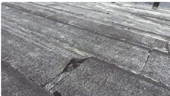
Photo showing scrim showing through deteriorated roof.
