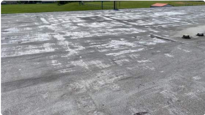
Photo showing scrim showing through deteriorated roof.
