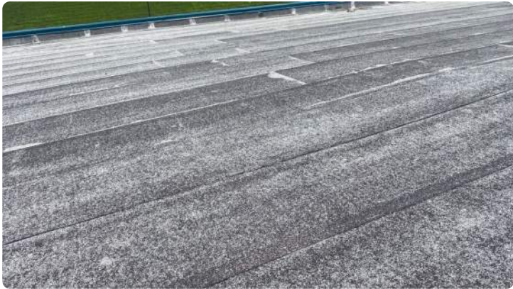
Photo showing deteriorated field with exposed scrim.
