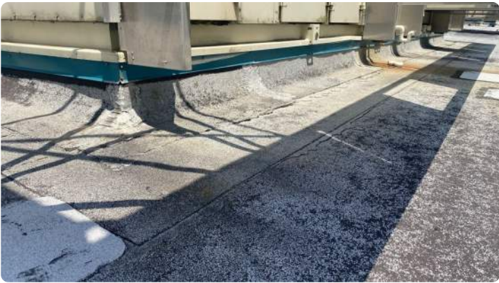
Photo showing condition of the projection flashings.
