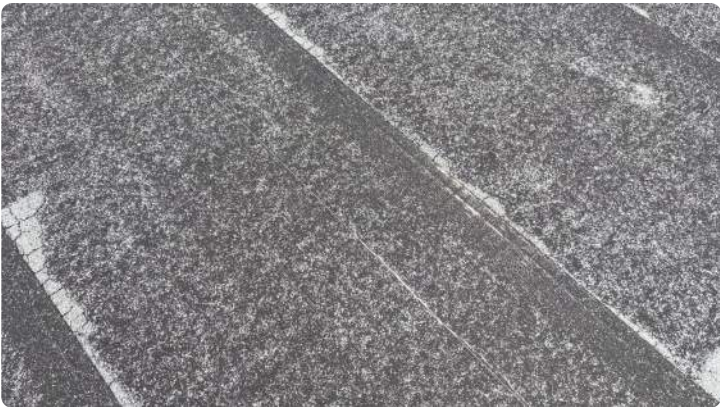
Photo showing additional skim exposed at seams.
