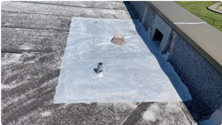
Photo showing aluminum coating around drain.
