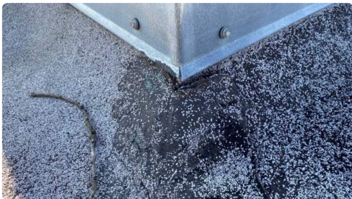
Photo showing deteriorating projection flashings.
