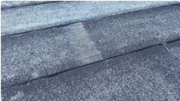
Photo showing scrim visible through the deteriorating field.
