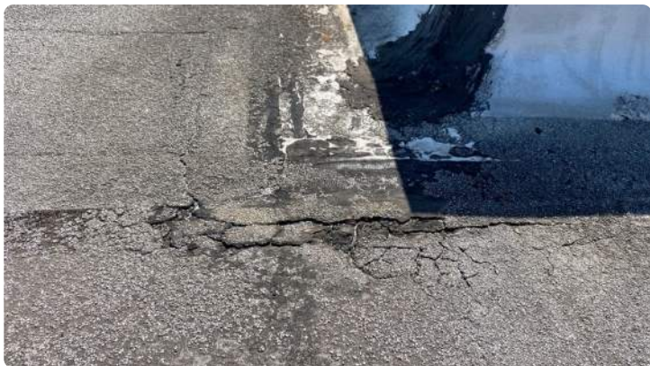
Photo showing alligatoring in the projection flashings.
