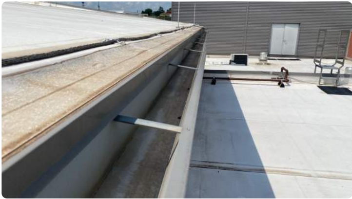
Photo showing condition of the gutter edge.
