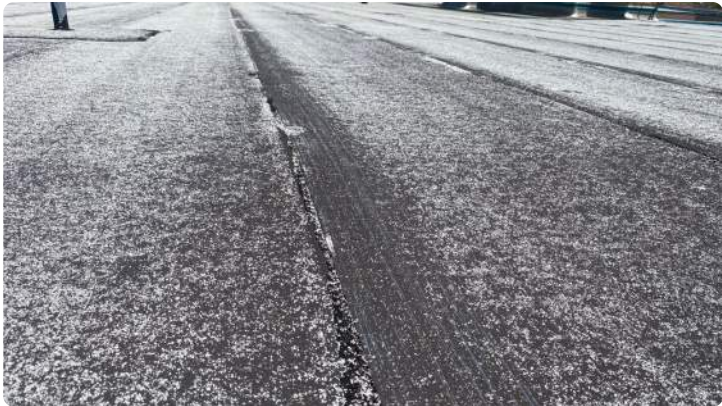
Photo showing addition deterioration in field.
