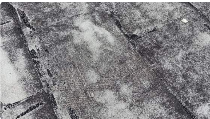
Photo showing skrim visible through the deteriorated field.
