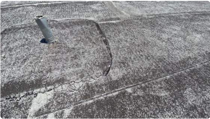
Photo showing deteriorating field.
