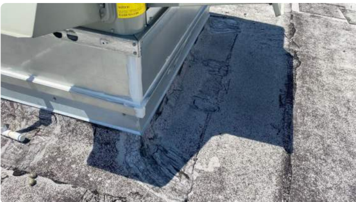
Photo showing cracking in projection flashings.
