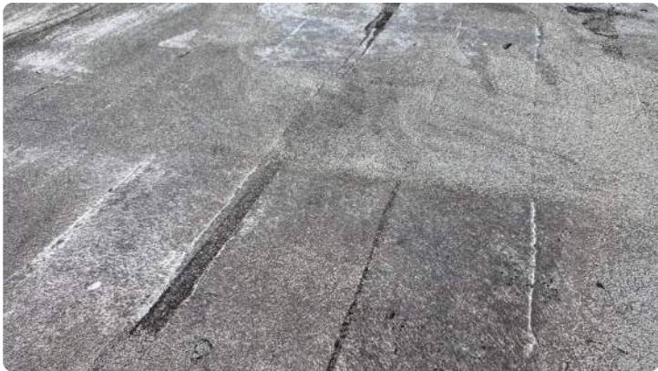
Photo showing scrim showing through deteriorated roof.
