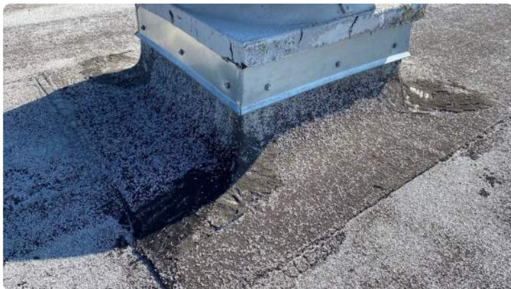
Photo showing condition of the projection flashings.
