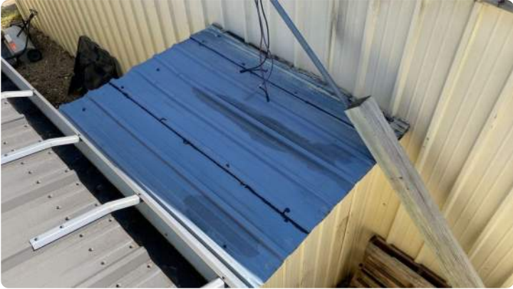
Photo showing condition of adjacent metal roof.
