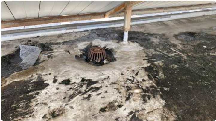
Photo showing coating deteriorating around drain.
