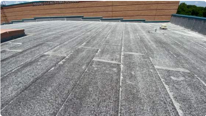
Photo showing deteriorated field.
