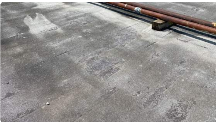
Photo showing skim showing through deteriorated roof.
