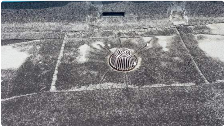
Photo showing deterioration around drain.
