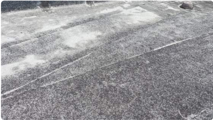
Photo showing loose granules and deterioration of field.
