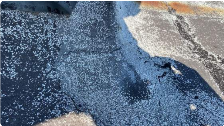
Photo showing cracking and deteriorating projection flashings.
