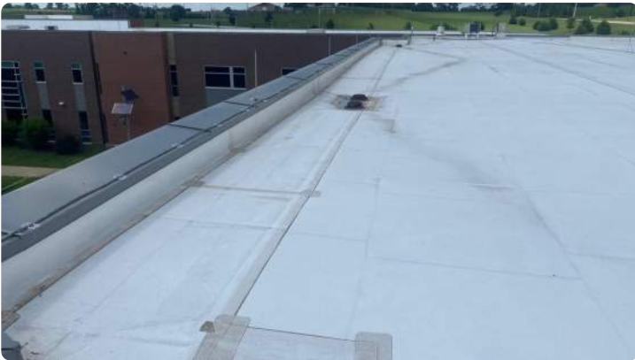
Photo showing condition of perimeter flashings.
