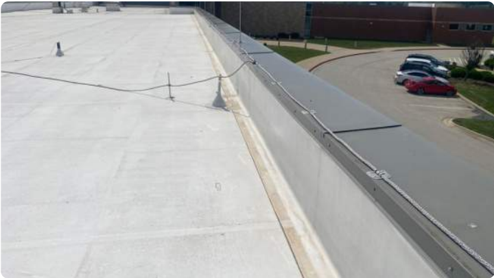
Photo showing condition of perimeter flashings.
