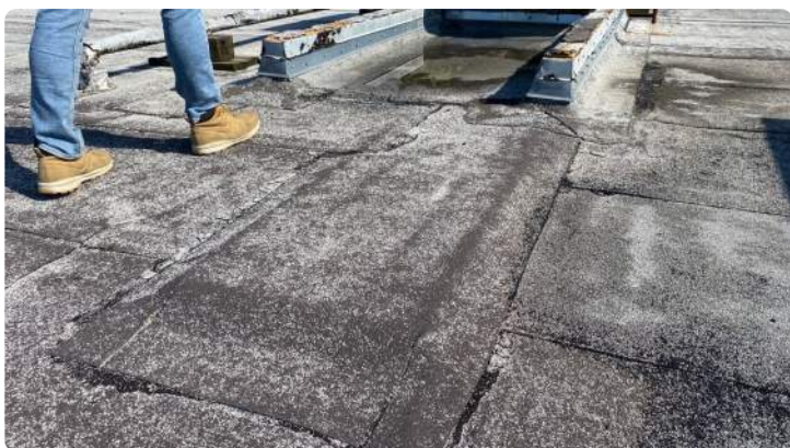
Photo showing deteriorating field.
