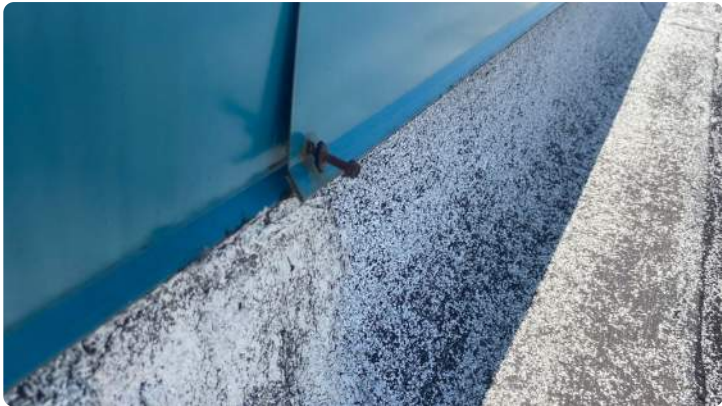
Photo showing screw backing out of the metal perimeter cap.
