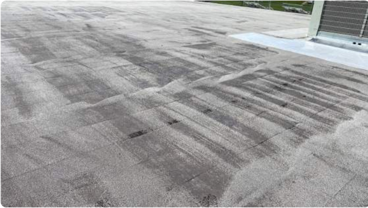
Photo showing scrim showing through deteriorated roof.
