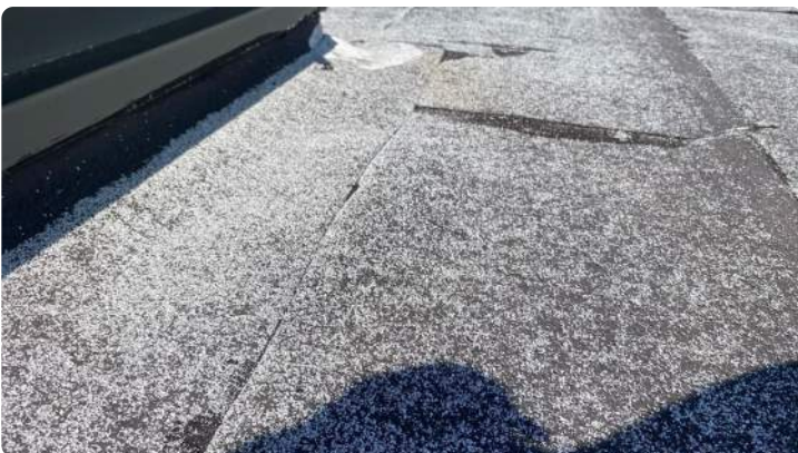
Photo showing blistering in the field.
