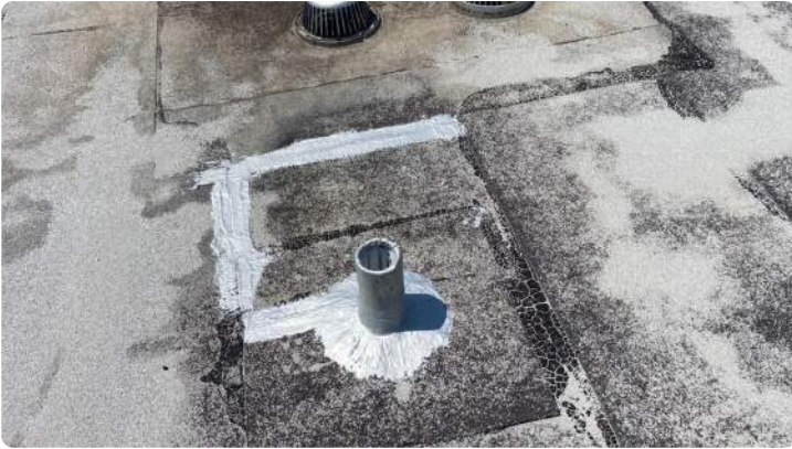
Photo showing aluminum coated seams on deteriorated field.
