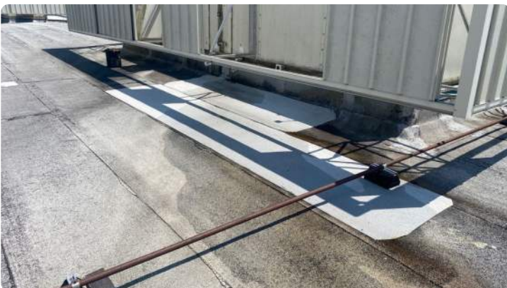
Photo showing patch previously made next to unit where condensation is ponding.
