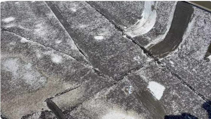
Photo showing blistering in deteriorated field.
