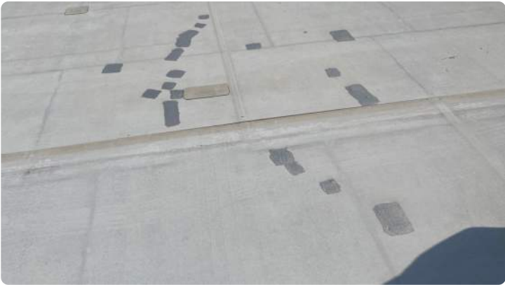
Photo showing multiple patches from previous damage.
