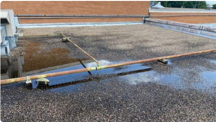
Photo showing additional ponding water.
