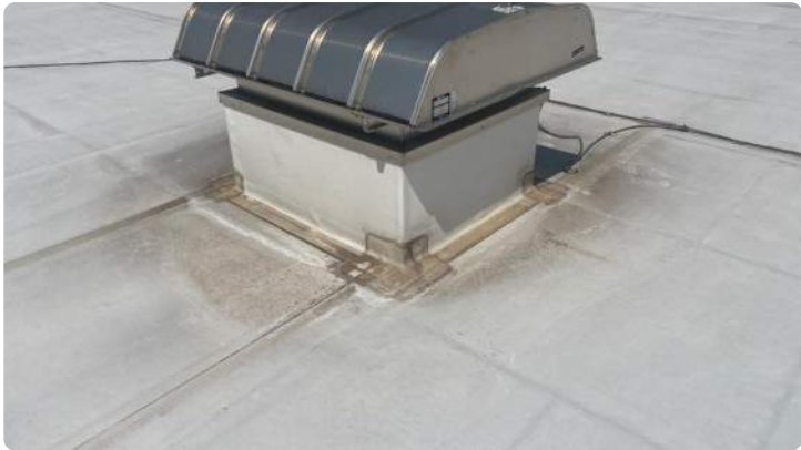
Photo showing condition of the projection flashings.
