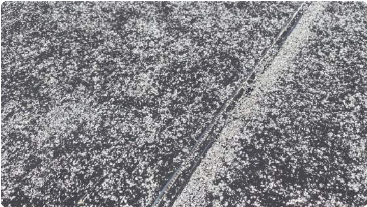
Photo showing scrim visible through deteriorating field.
