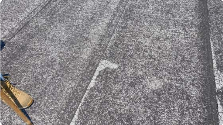
Photo showing deterioration of the field.
