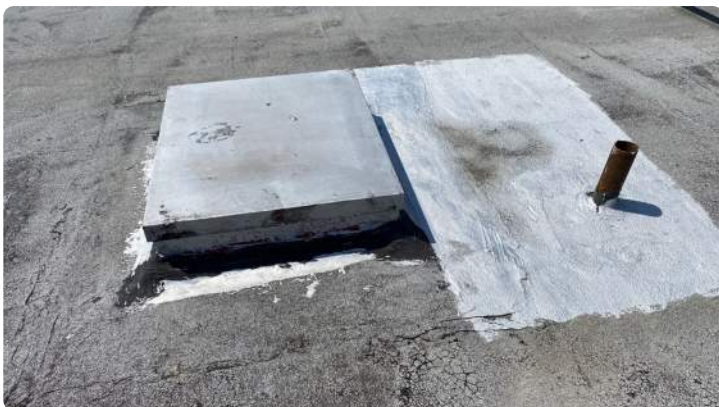
Photo showing additional area with aluminum coating.
