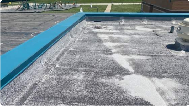
Photo showing granules piled up from deterioration.
