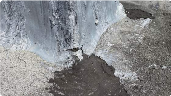
Photo showing deteriorating projection flashings.
