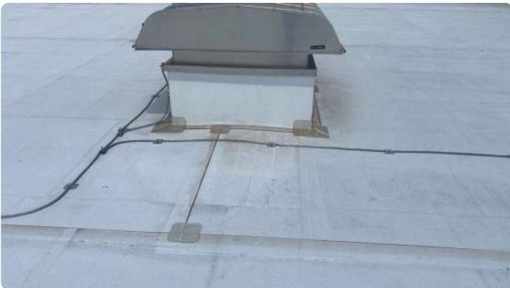
Photo showing condition of the projection flashings.
