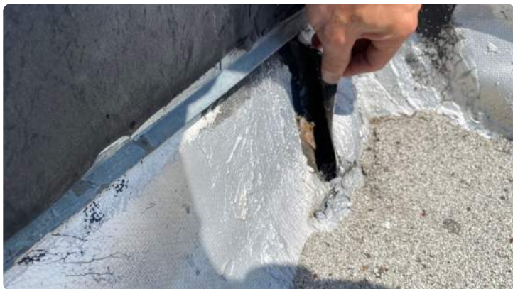
Photo showing flashings pulling loose.
