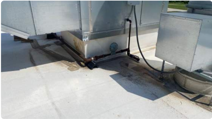
Photo showing condition if the projection flashings.
