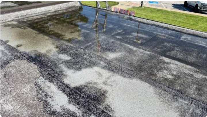
Photo showing ponding water along perimeter.
