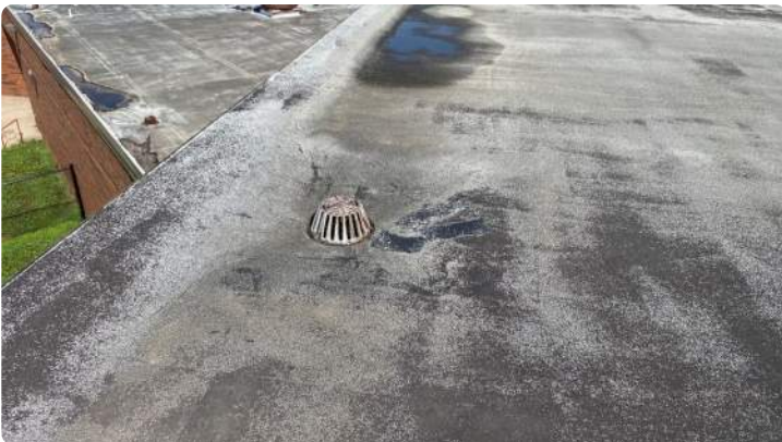
Photo showing condition of the drain.
