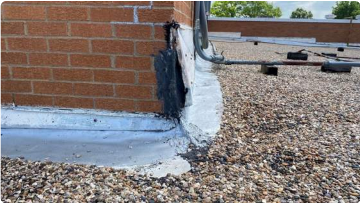
Photo showing a corner flashing that is beginning to open up.
