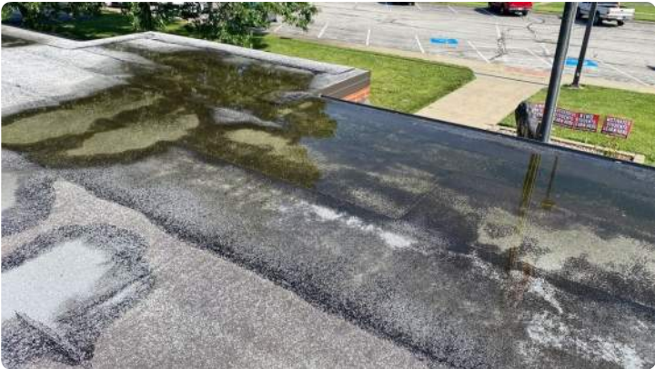
Photo showing ponding water along perimeter.
