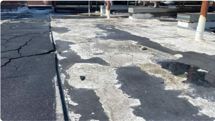
Cover board pushing up
