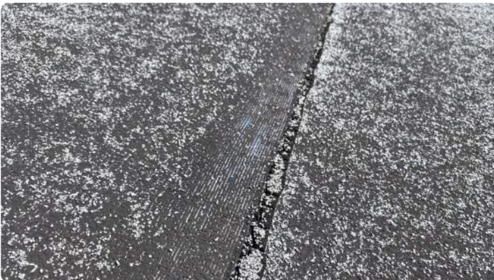
Photo showing scrim showing through deteriorated roof.
