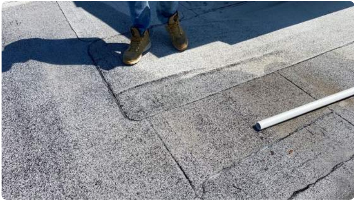
Photo showing blistering near condensate pipe.
