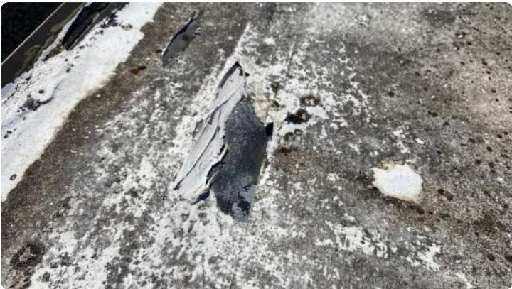
Photo showing deteriorating coating.
