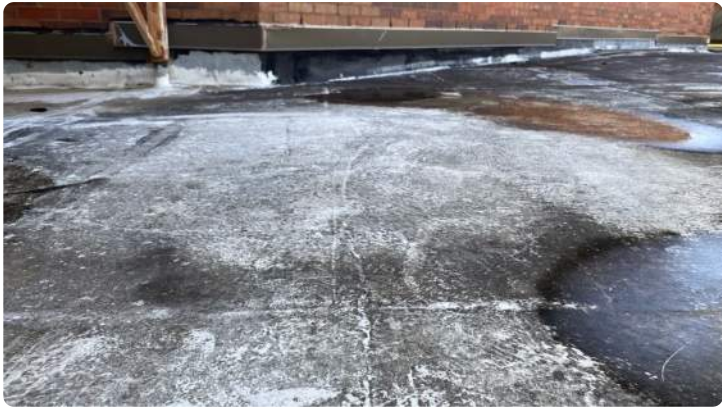
Cover board pushing up
