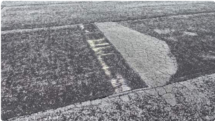
Photo showing exposed scrim at seam.
