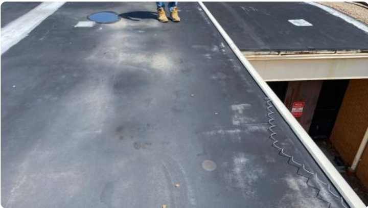
Photo showing area of EPDM pushing up.
