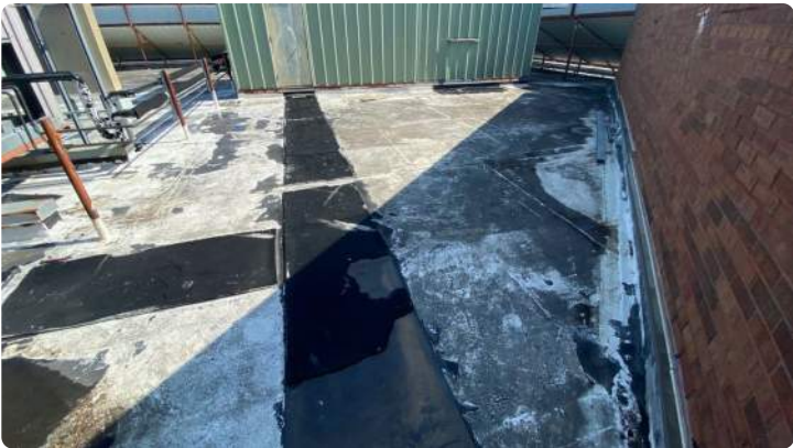
Photo showing area with loose membrane.
