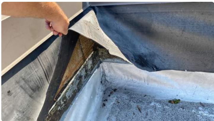
Photo showing loose perimeter flashing.
