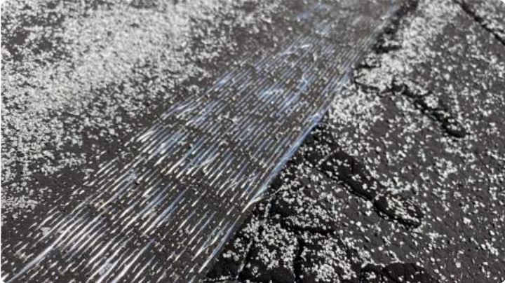
Additional photo showing skim showing through deteriorated roof.
