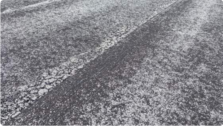
Photo showing deterioration of field.
