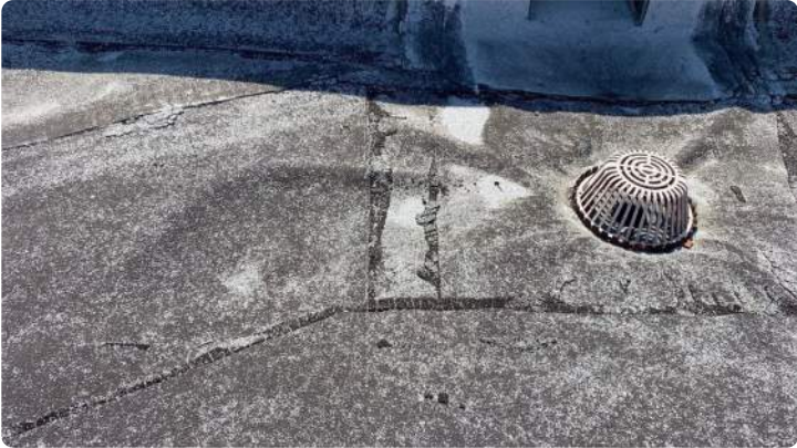
Photo showing wrinkles around drain and deteriorated field.
