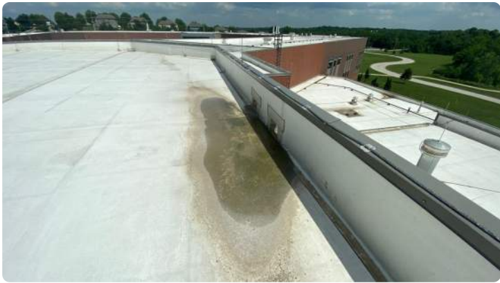
Photo showing condition of perimeter flashings.
