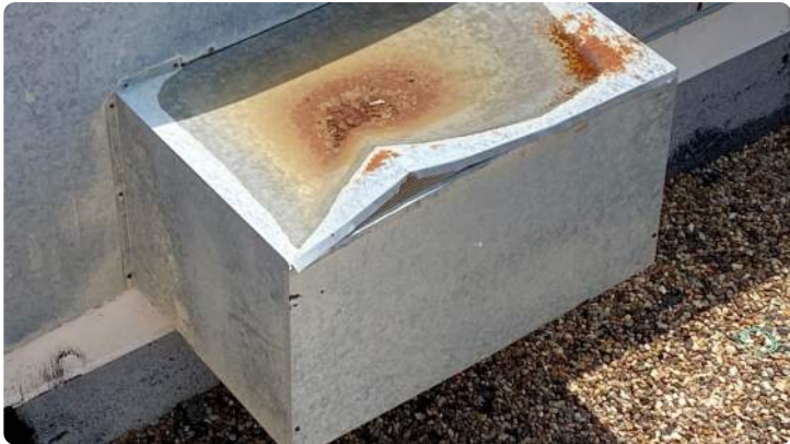
Photo showing ductwork with damaged wall open to elements.
