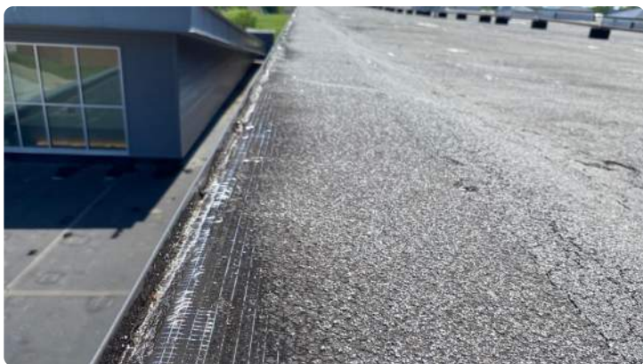
Photo showing skim showing through deteriorated roof at perimeter.
