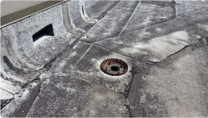
Photo showing missing drain strainer.
