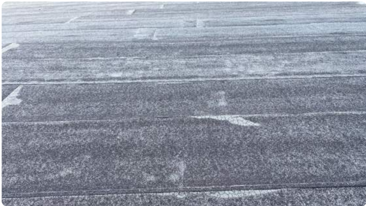
Photo showing deterioration in field.
