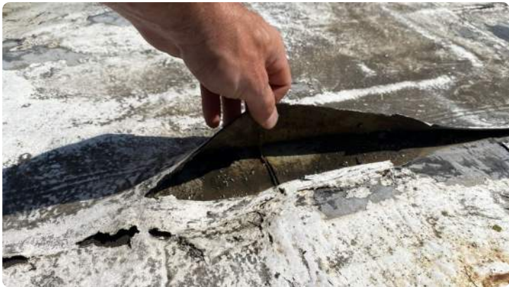
Photo showing a seam pulling loose.
