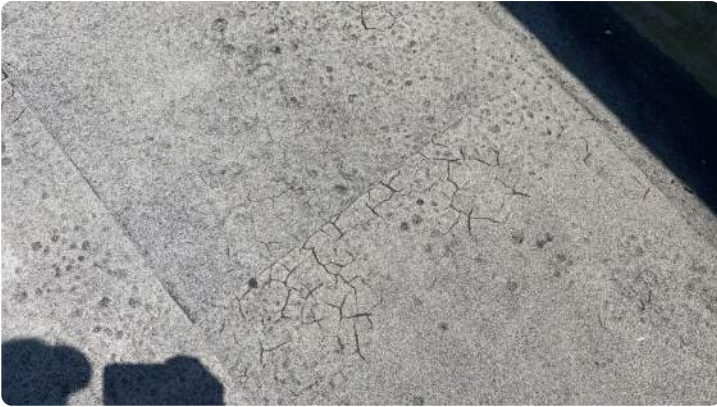
Photo showing additional cracking in field.
