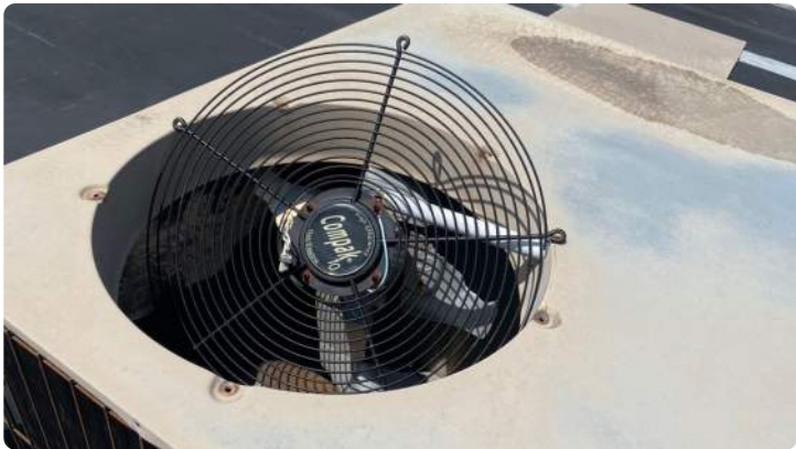
Photo showing fan on HVAC unit that is dislodged.
