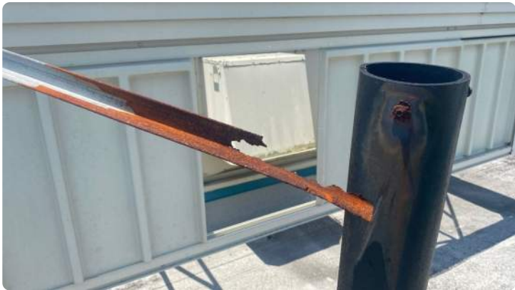
Photo showing rusted vent stack supports.
