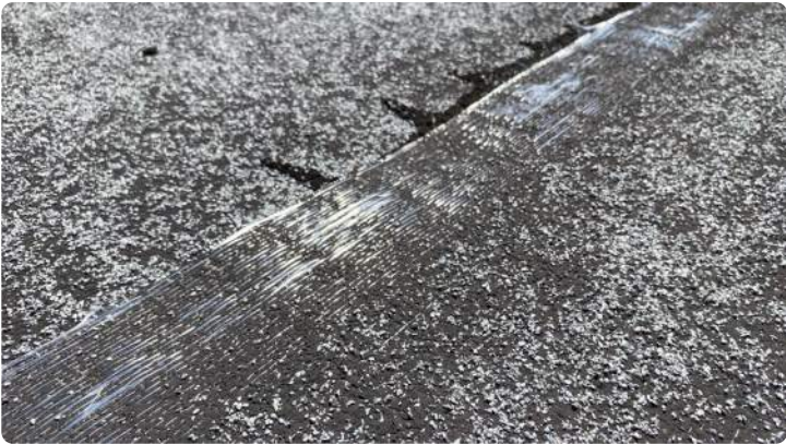
Photo showing skrim showing through deteriorated roof.
