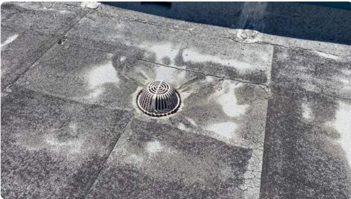
Photo showing blistering and granules piled up around drain.
