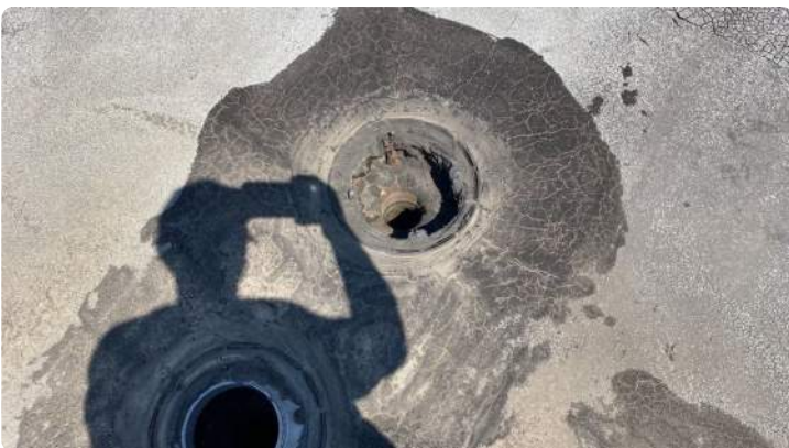
Photo showing condition of the drain missing a strainer.
