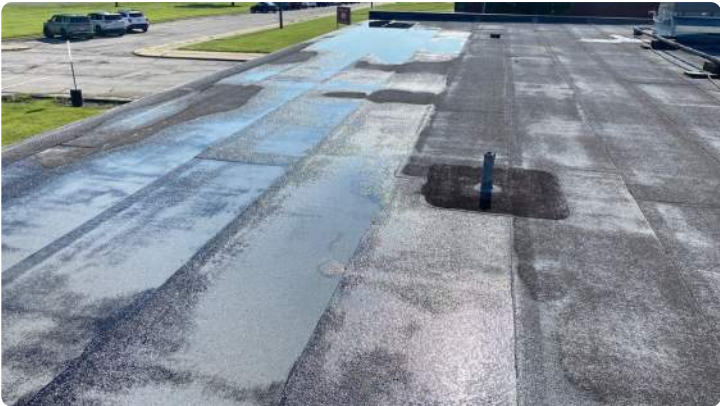
Photo showing additional ponding water.
