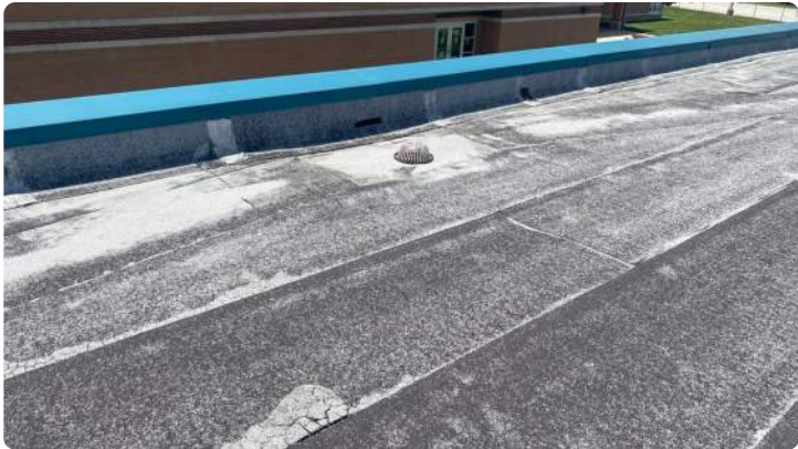
Photo showing granules piled up along drain valley and in drain.
