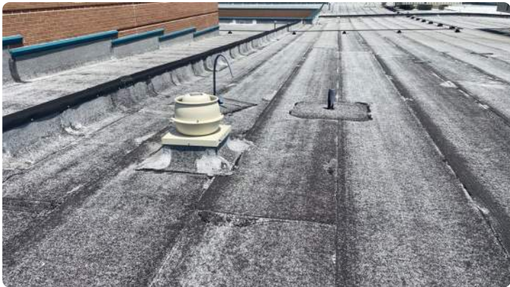
Photo showing roof with granules deteriorated from field.
