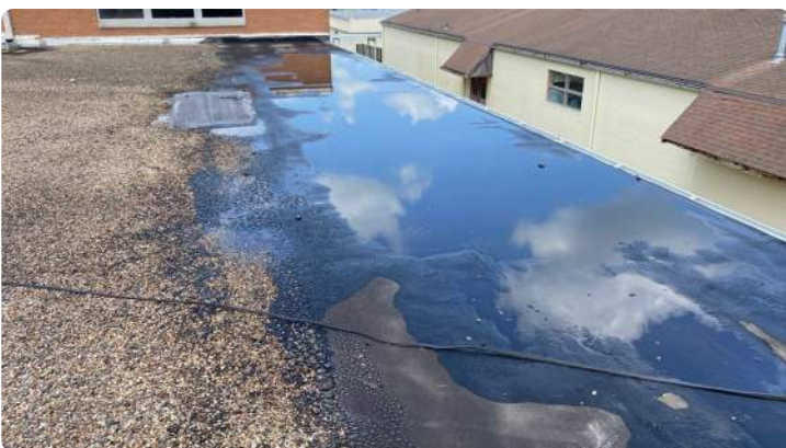
Photo showing ponding water.
