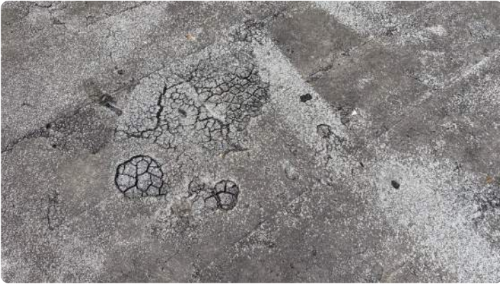
Photo showing alligatoring in field.
