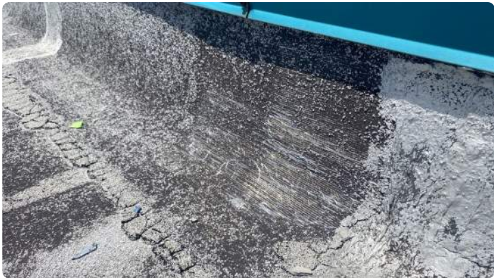
Photo showing skim visible through deteriorating perimeter.
