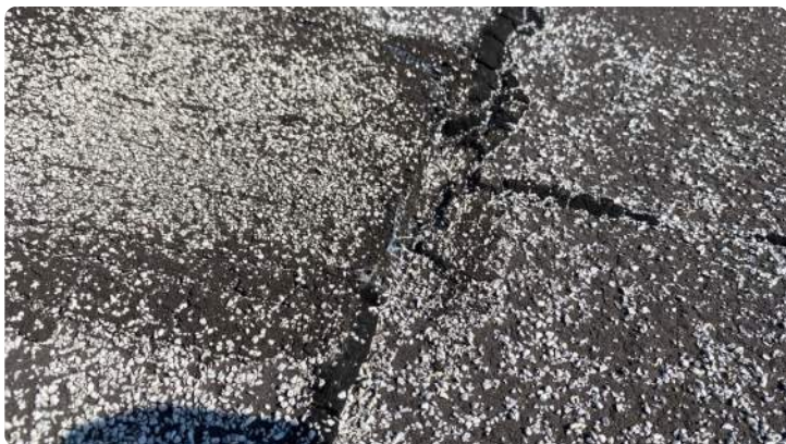
Photo showing skim exposed in deteriorating field.
