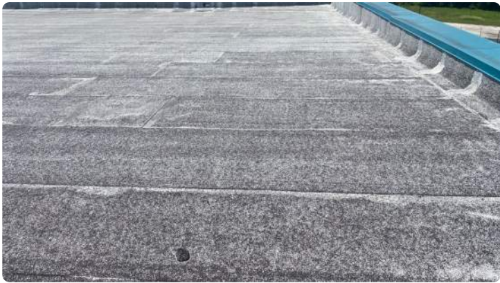
Photo showing skim visible through deteriorating field.
