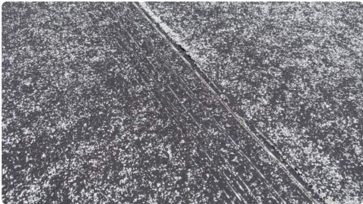
Photo showing skim showing through field at seam.
