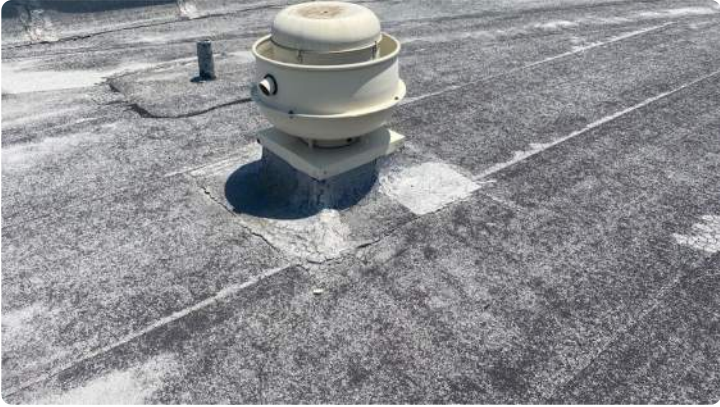
Photo showing condition of the projection flashings and deteriorated field.
