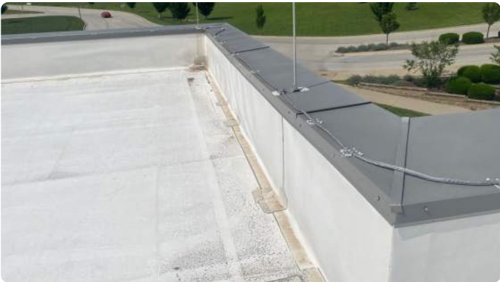
Photo showing condition of perimeter flashings.
