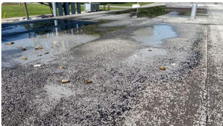
Photo showing ponding water.
