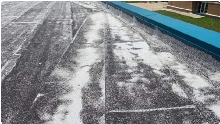
Photo showing granules piled up from deterioration.
