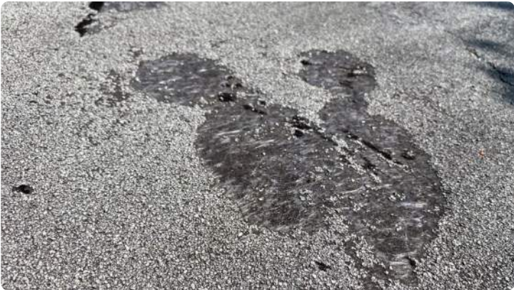
Photo showing skim showing through deteriorated roof.
