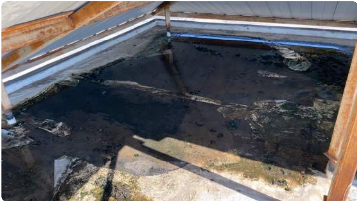
Photo showing ponding water under awning.
