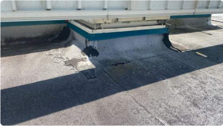
Photo showing condition of the projection flashings.
