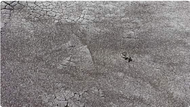
Photo showing alligatoring and a hole in the field.
