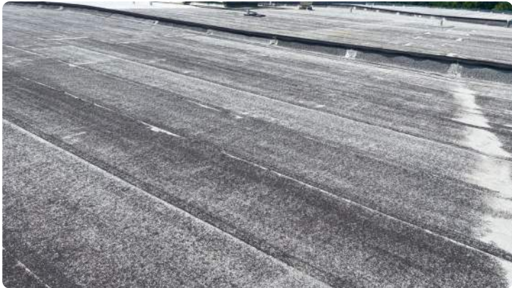
Photo showing additional skim exposed and deterioration in field.
