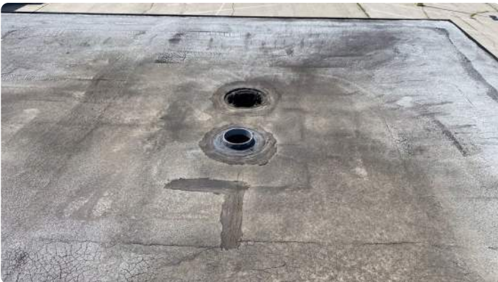
Photo showing drain with and overflow drain cap.
