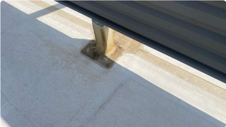
Photo showing condition if the projection flashings.
