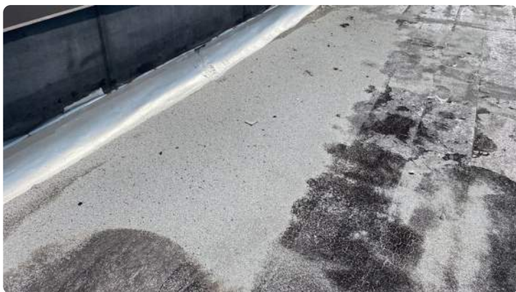
Photo showing loose granules from deteriorating roof piling up.
