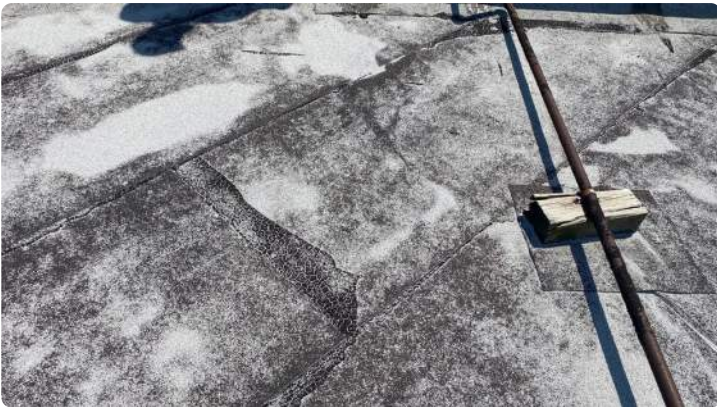
Photo showing granules piled up and deterioration of the field.
