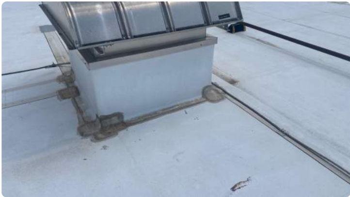
Photo showing condition of the projection flashings.
