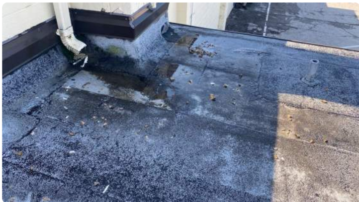
Photo showing deteriorating field.
