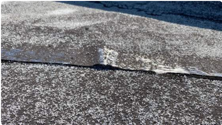
Photo showing a fishmouth in the deteriorated field and blistering.
