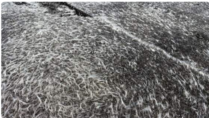
Photo showing scrim showing through deteriorated roof.
