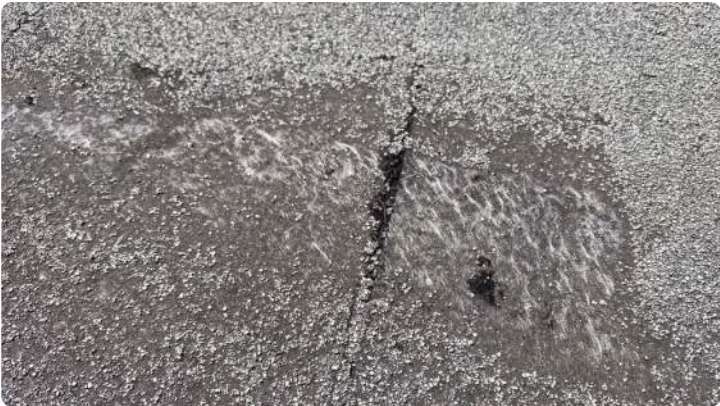
Photo showing scrim showing through deteriorated roof.
