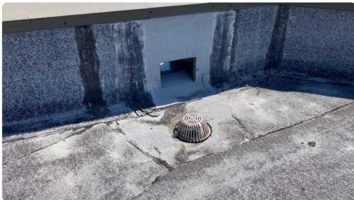
Photo showing granules from deteriorated roof piling up around drain.
