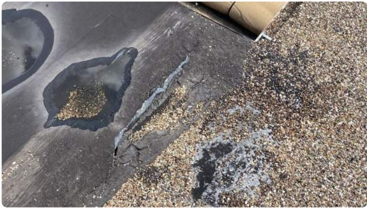
Photo showing area coated in roofing mastic beginning to crack.
