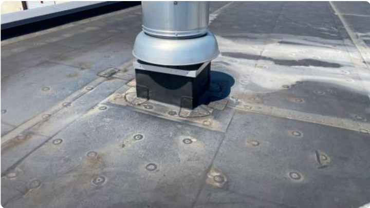
Photo showing condition of the projection flashings.
