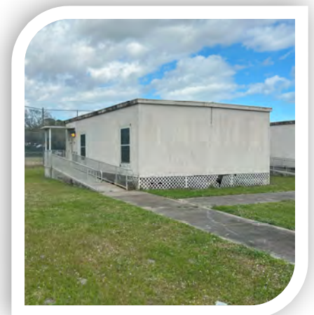
Southwest Middle School Surplus Relocatable in poor condition, Recommended for DCR and demolition.
