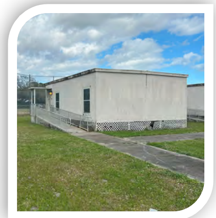
Southwest Middle School Surplus Relocatable in poor condition, Recommended for DCR and demolition.
