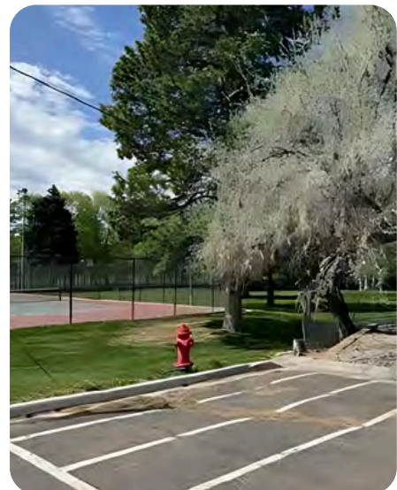
Park Fire Hydrant
