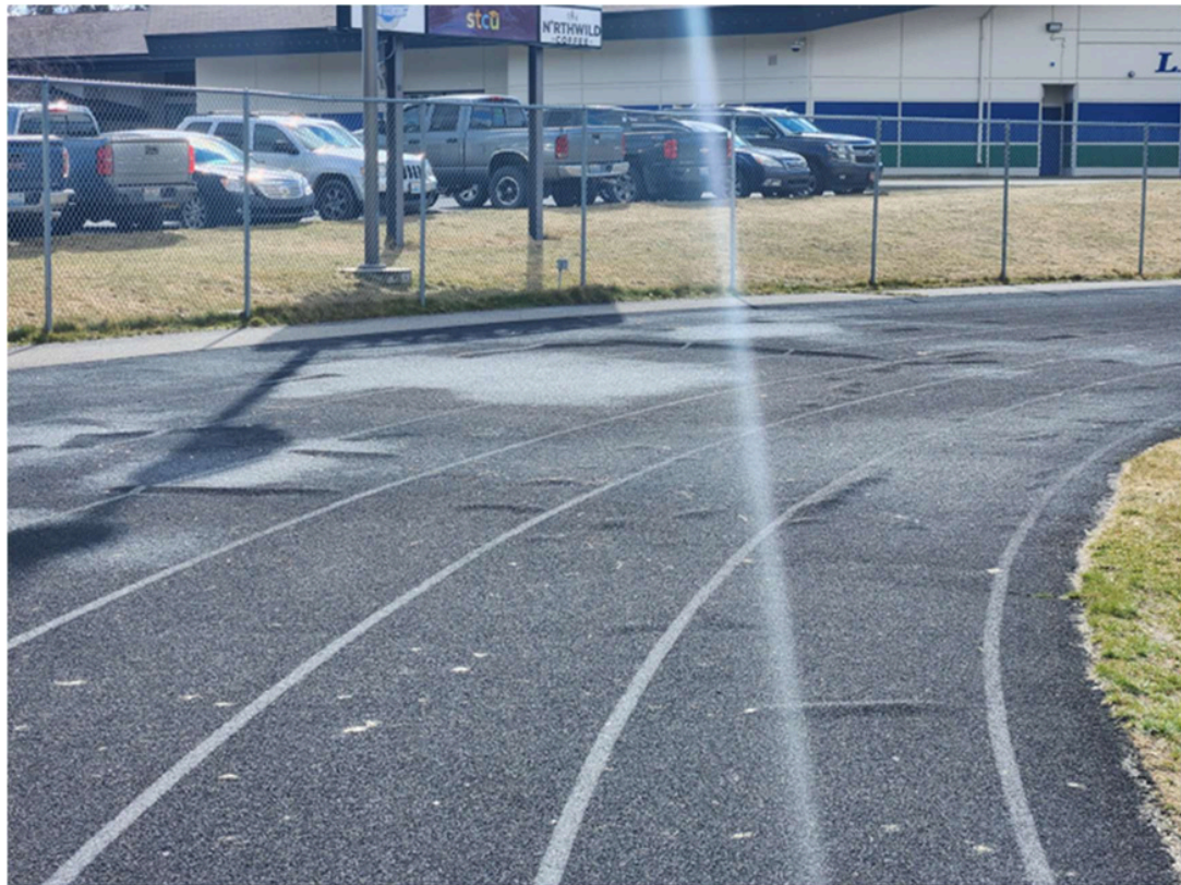
LHS track has extensive cracking and is delaminating from the asphalt surface
