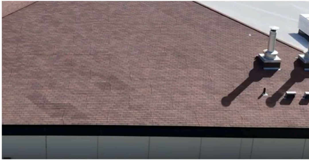
LHS roof continues to fail and needs to be replaced
