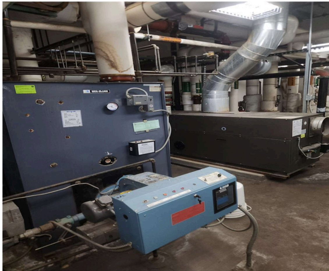
Original LHS boilers from 1990 - only one is operational
