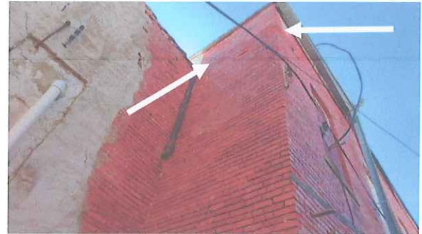
NORTHEASTERN EXTERIOR WALL MOVEMENT
