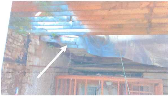
REAR OVERBUILT STRUCTURE FLOOR FAILURE
