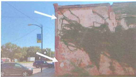
WESTERN WALL MOVEMENT NEXT TO NORTHERN WALL
