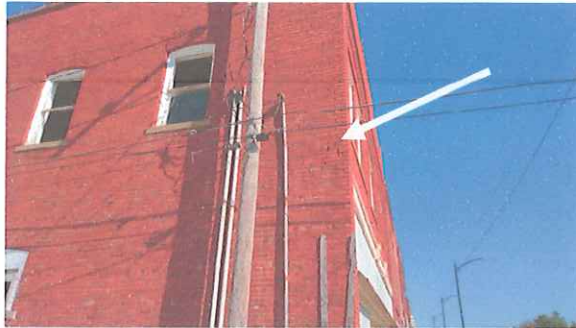
SOUTHWESTERN EXTERIOR WALL MOVEMENT
