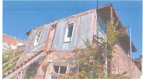
OVERBUILD ON THE REAR SINGLE STORY ADDITION
