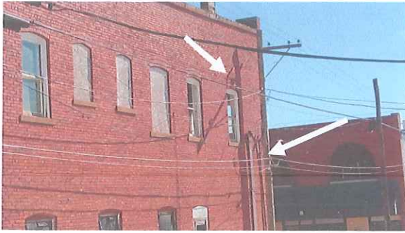
SOUTHWESTERN EXTERIOR WALL MOVEMENT
