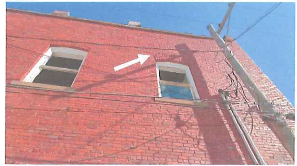
SOUTHWESTERN EXTERIOR WALL MOVEMENT
