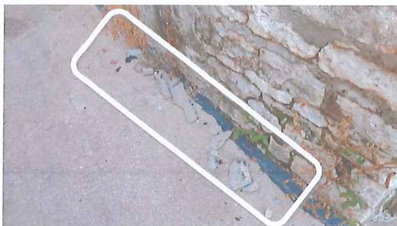
FALLING DEBRIS INDICATIONS
