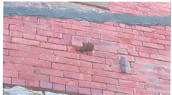
FAILING EXTERIOR BRICK VENEER
