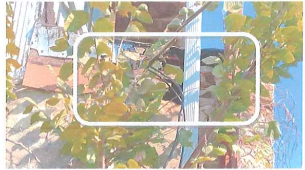
REAR OVERBUILT STRUCTURE FLOOR CONDITION
