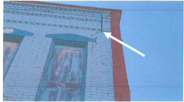
NORTHERN WALL CRACKING NEXT TO WESTERN WALL
