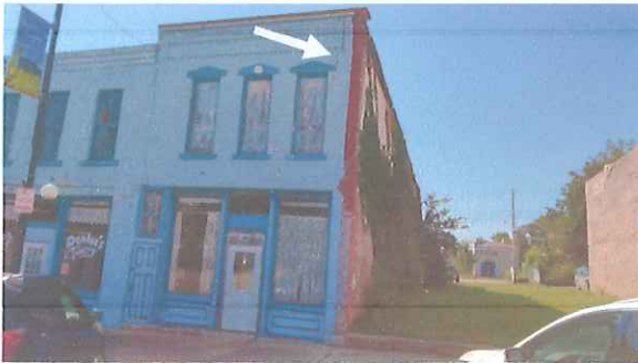
NORTHERN WALL MOVEMENT NEXT TO WESTERN WALL
