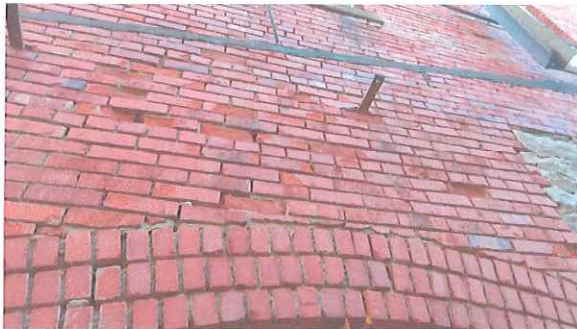
TYPICAL FAILING BRICK FACE SHELLS
