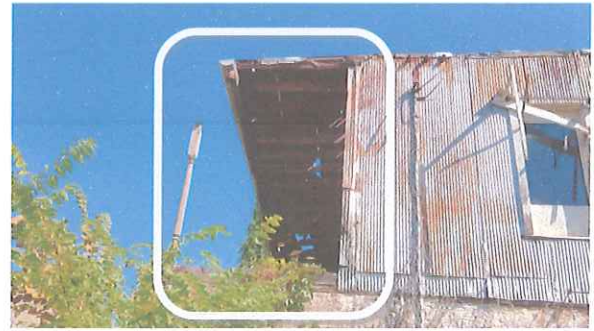
REAR OVERBUILT STRUCTURE DETERIORATION
