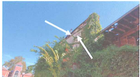
WESTERN WALL CRACKING/MOVEMENT
