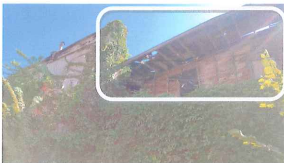
REAR OVERBUILT STRUCTURE DETERIORATION
