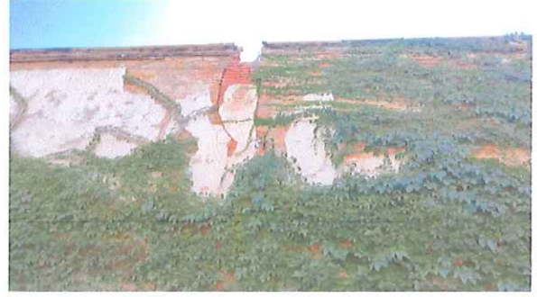
WESTERN WALL CRACKING/MOVEMENT
