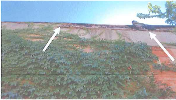
WESTERN WALL CRACKING/MOVEMENT
