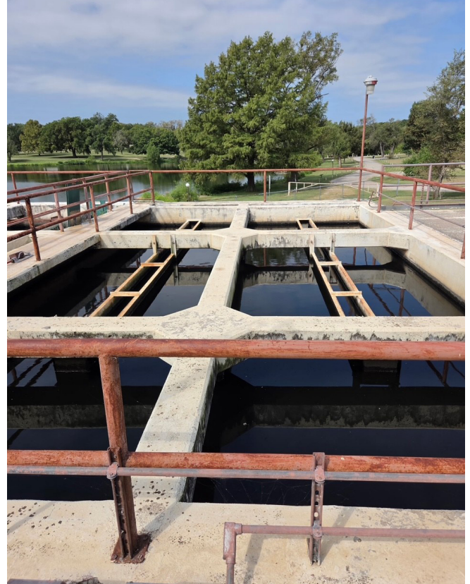
GARNETT WATER TREATMENT PLANT
