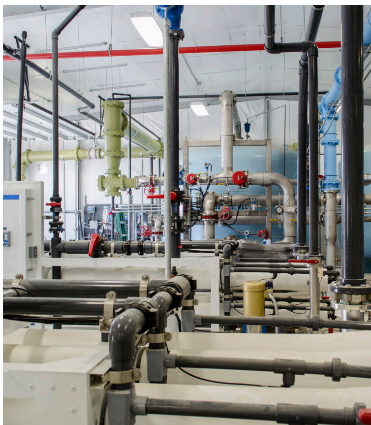
PWWSD #26 TREATMENT TOWER AND WATER MAIN
