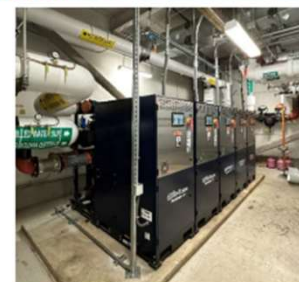
GSHP recently installed at Salem State University
