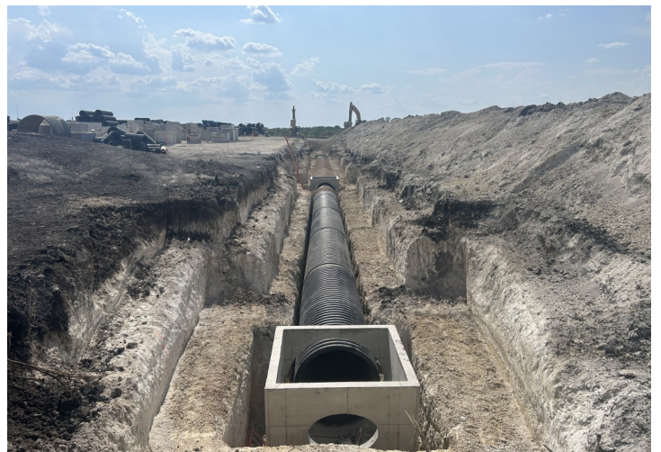
Pond A - Storm Line
