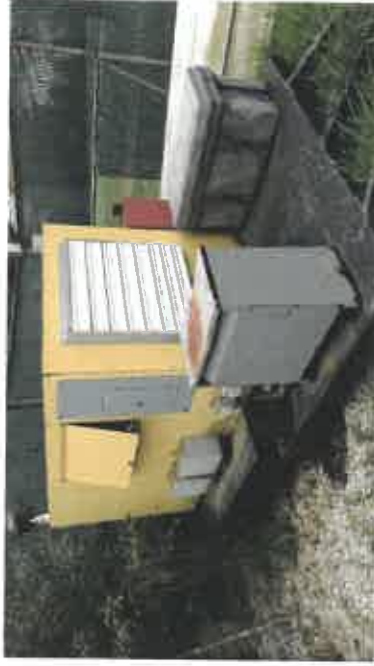
Stand By Generator trailer mounted, 6 cylinder, motor runs, 3 phase, one phase does not work. Minimum Bid $250
