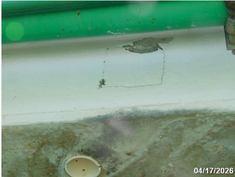
Photo 3: Spalled and Delaminated grout patch for the transverse post tension rod in the south face of Slab Unit 9-7
