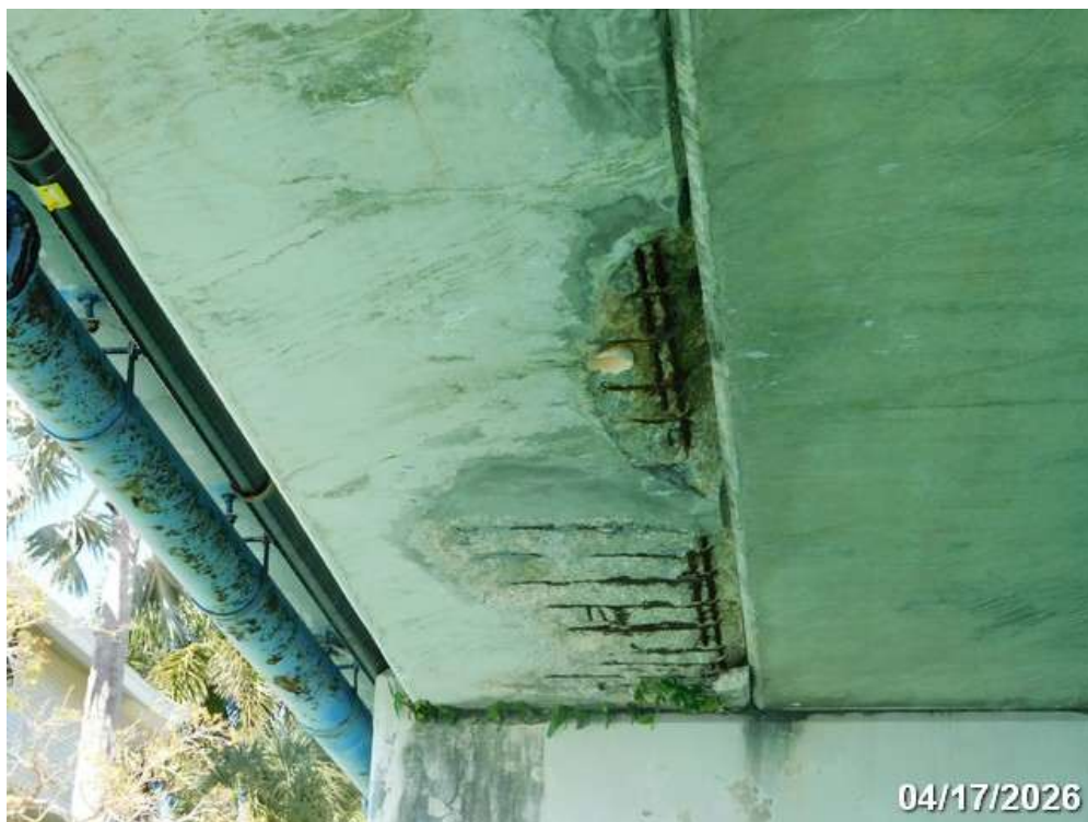
Photo 2: General view and close up of spall/delamination at Slab Unit 9-1 at midspan.
