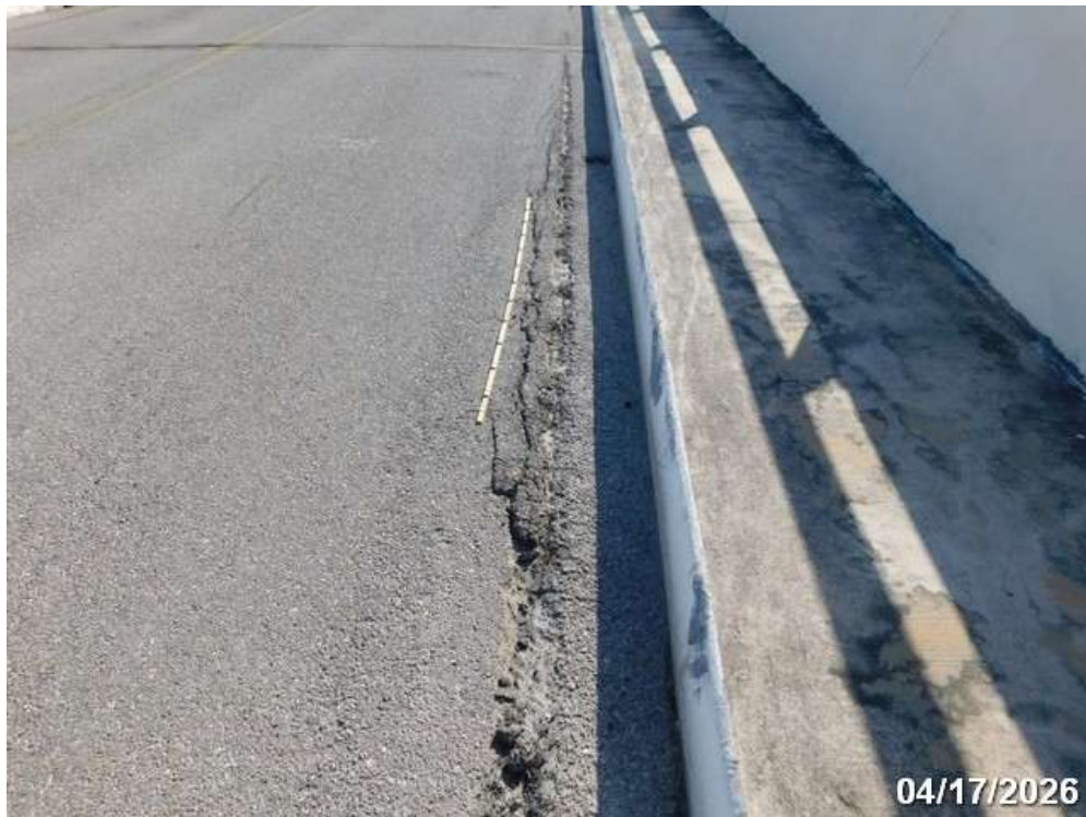
Photo 4: Crack with upheaving in the asphalt over Slab Units 9-1 and 9-2 joint. FDOTTampaBay.com | @MyFDOT_Tampa | Facebook.com/MyFDOTTampa
