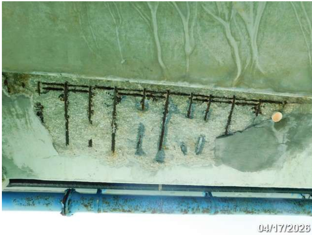
Photo 1: General view of spall/delamination at Slab Unit 9-1 starting at Bent 9.
