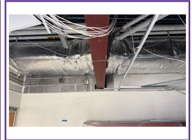
Administrative Office Duct
