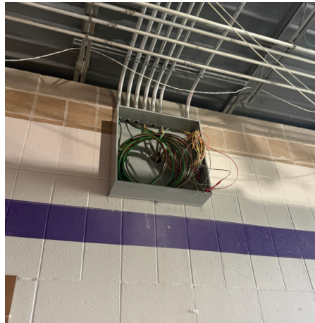
Junction Box Area D
