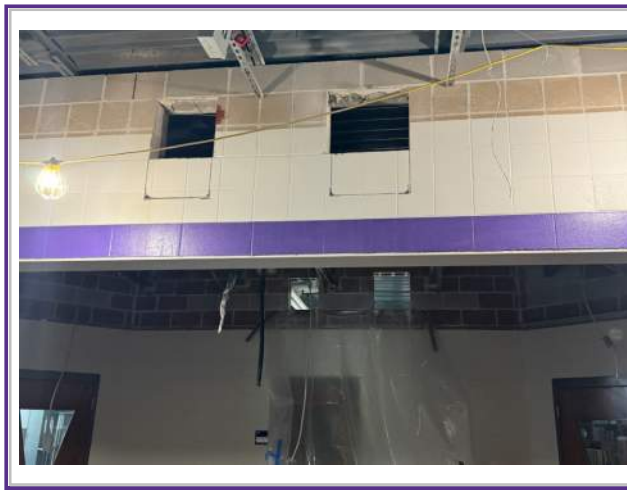
Finecut duct penetrations
