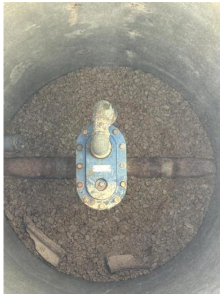
The Bloomington Well air valve, as found: not plumbed above grade and open to the manhole environment.
