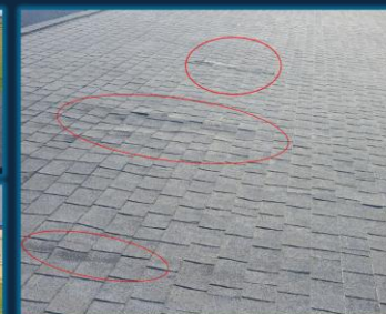
Buckling of the shingles
